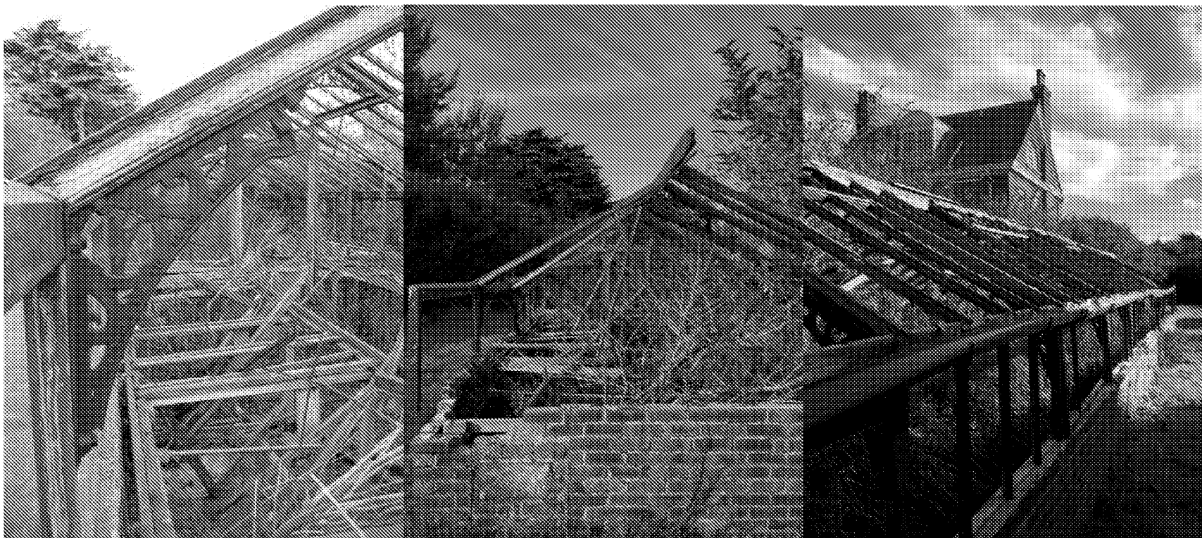
FIG . 29 - PBA PHOTO MONTAGE - DERELICT GLASSHOUSE
