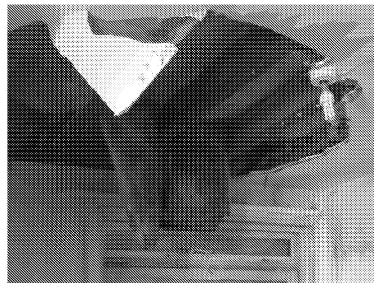
FIG. 24 - PBA PHOTO - CEILING IN THE COTTAGE HAS COLLAPSED DUE TO WATER INGRESS RESULTING FROM LEAD FLASHING STOLEN FROM THE ROOF
