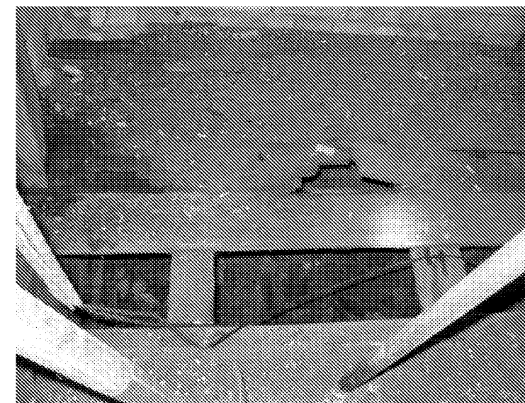
FIG. 25 - PBA PHOTO - LAUNDRY - ROTTEN FLOORBOARDS AT GROUND FLOOR LEVEL
