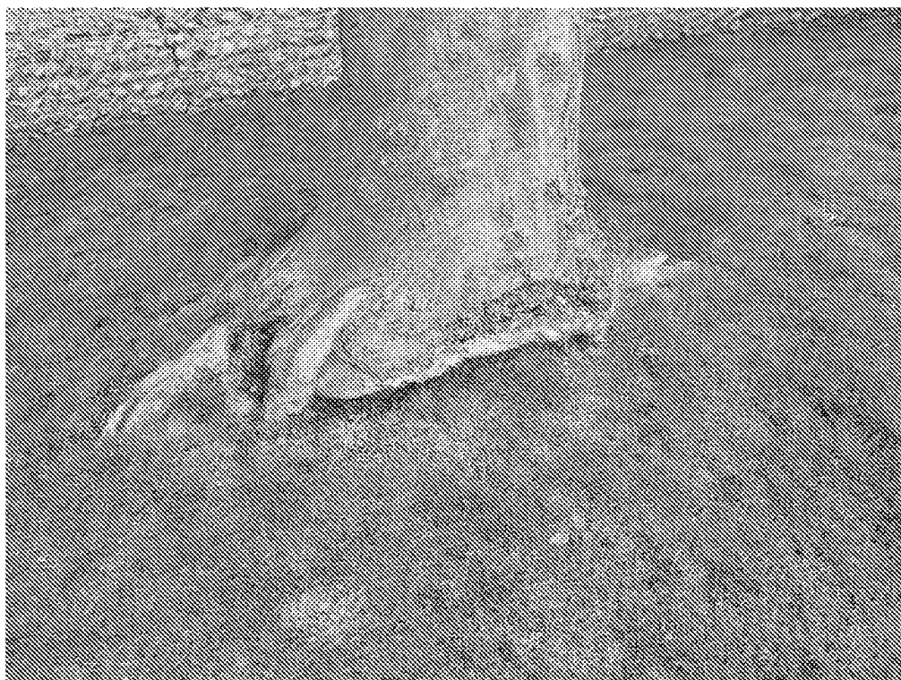
T4 Ash showing poor condition of buttress & roots
