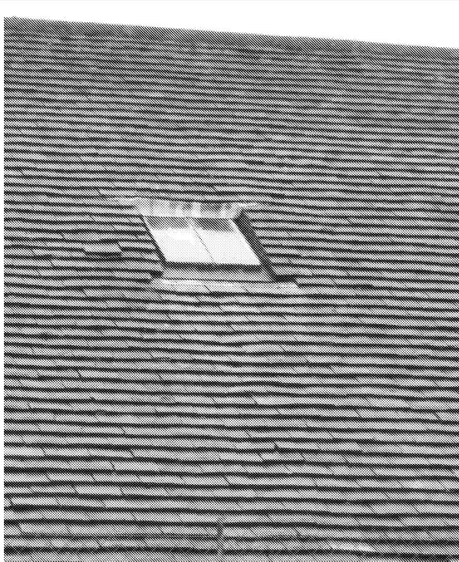
Photograph 8: Gaps under roof tiles on southern aspect of roof of main house.
