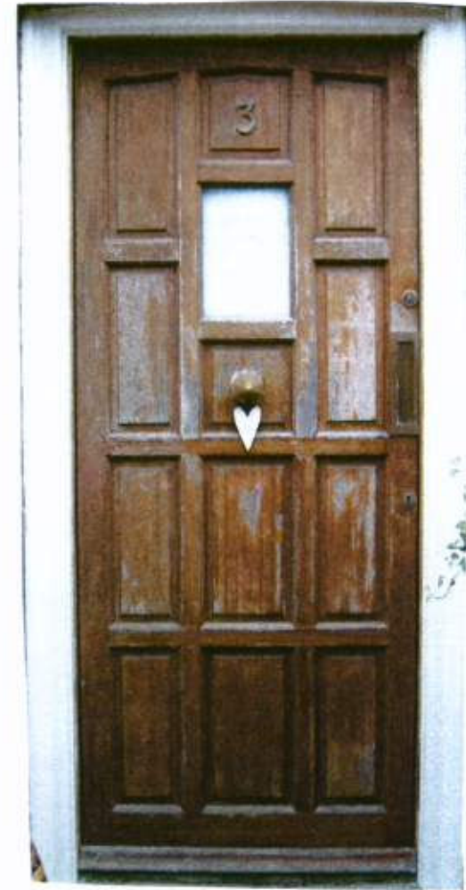
STYLE OF DOOR REMOVED
