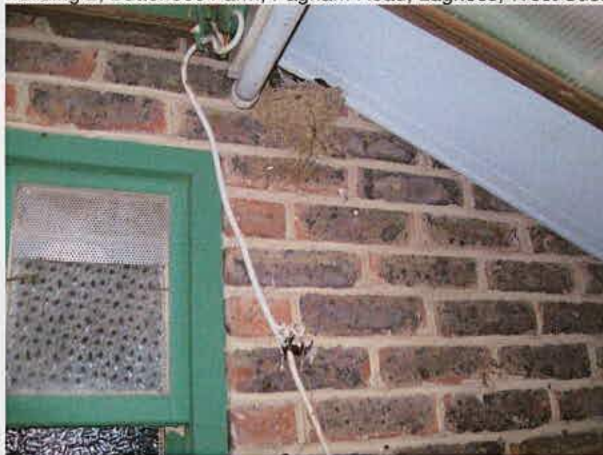
Photograph 4.2: Active Swallow nest, located in the 'lean to' at the south-west of Building 2, Butterlees Farm, Pagham Road, Lagness, West Sussex.
