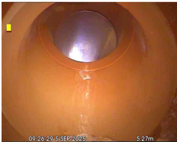
RESEVOIRX_10982a43-b268-4974-9c2a-bfa0fc3219ce_2025 0910_083715_578.jpg, 00:00:40, 5.14 m Line deviates up
