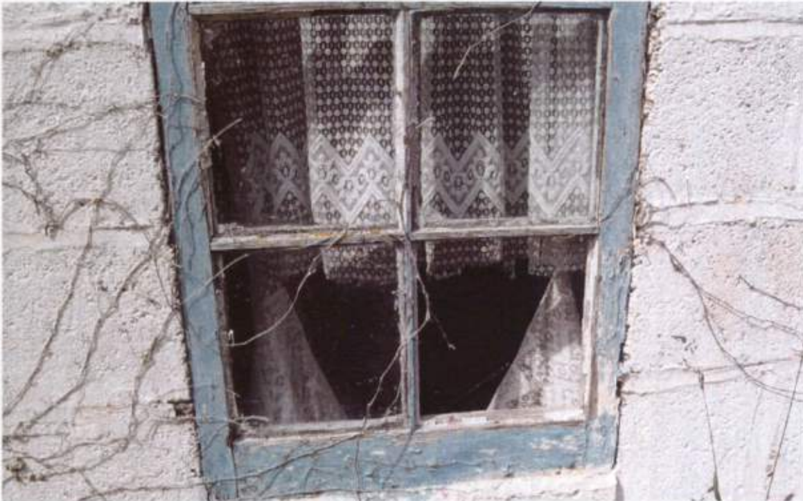
Photograph No. 9 - Broken panel allowing access to Nesting space within the Garage on Site. Opening is of a suitable size to allow Birds of either species to enter and exit.
