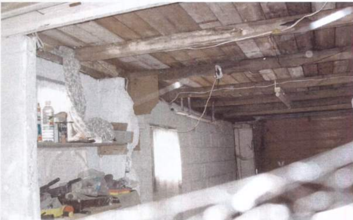
Photograph No. 10 - Potential space for Nesting Swallows found at juncture of Wall and Roof in Garage on Site. Potential space for Nesting Starlings on ledges found to the Northern end of Garage found on Site.
