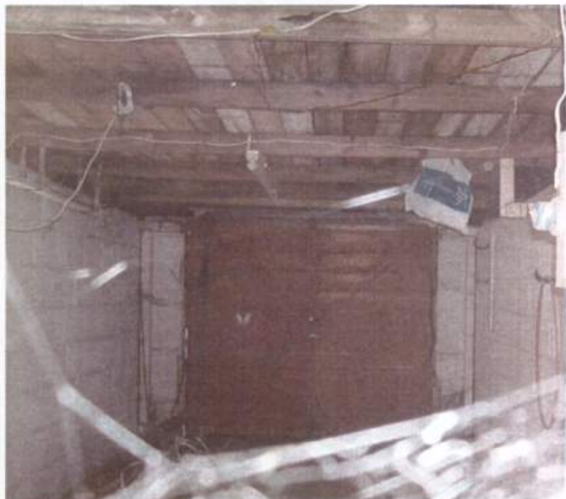
Photograph No. 11 - Potential space for Nesting Swallows found at juncture of Wall and Roof in Garage on Site. Potential space for Nesting Starlings on ledges found to the Northern end of Garage found on Site.
