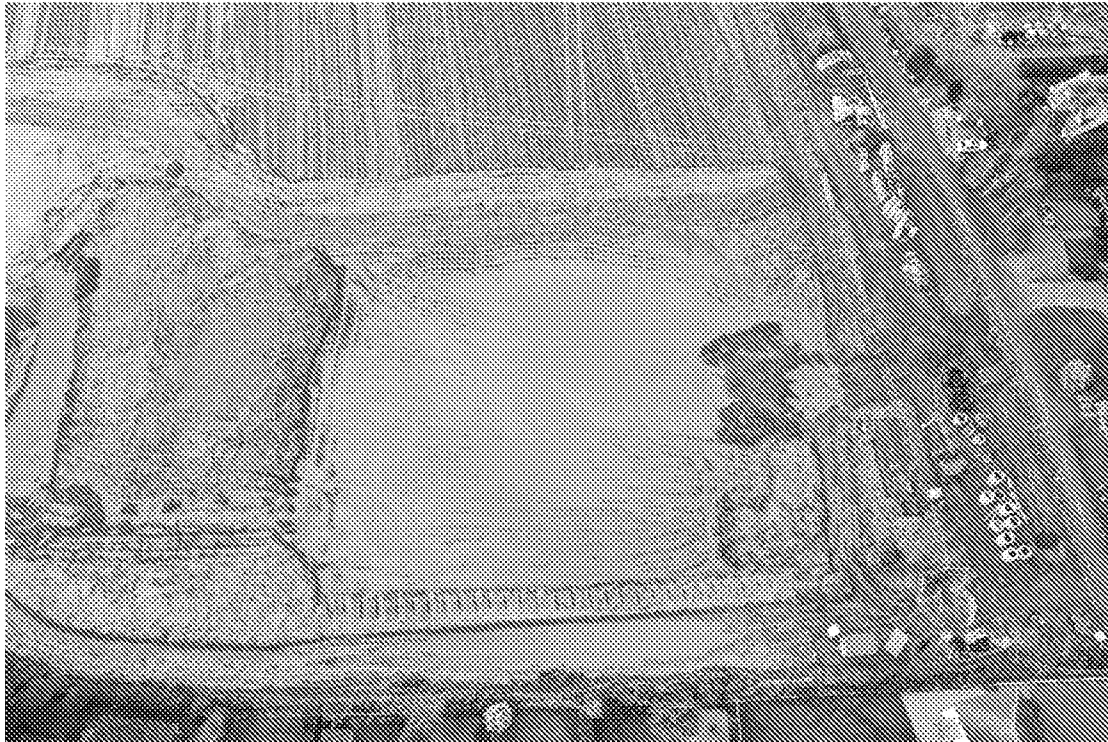
Photo 3. Taken 5/2/21. Indication that gardens of houses on Pagham Road are originally above level of deposition site. Note presence of blue asbestos decontamination wagon bottom right.
