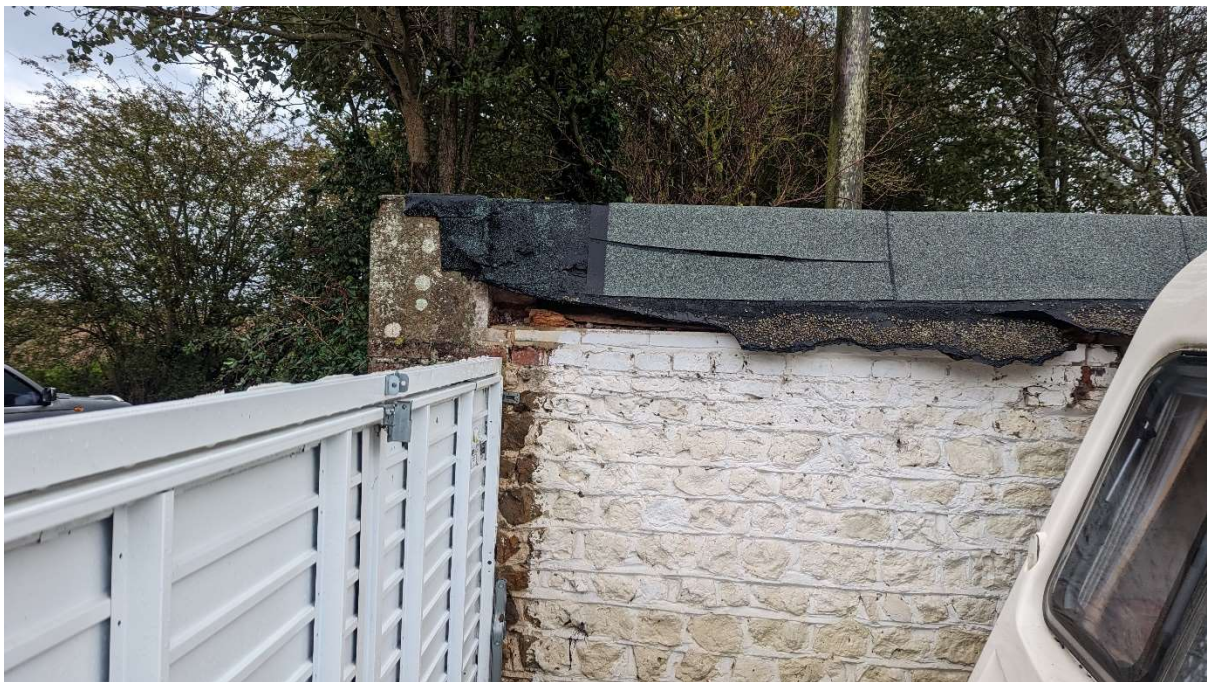
Photo 6 – View of the remains of the garage roof and door.
