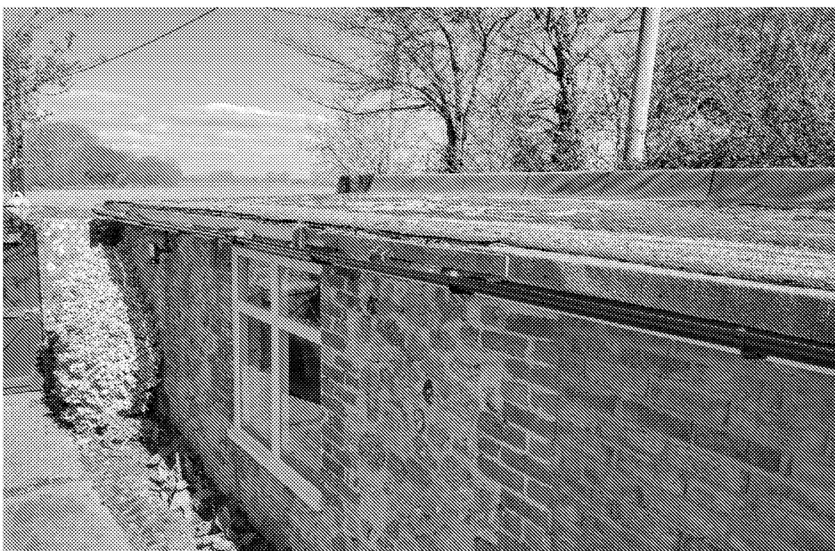
Plate VII : Grey Barn Garage – Roof in poor condition and suffering from water ingress
