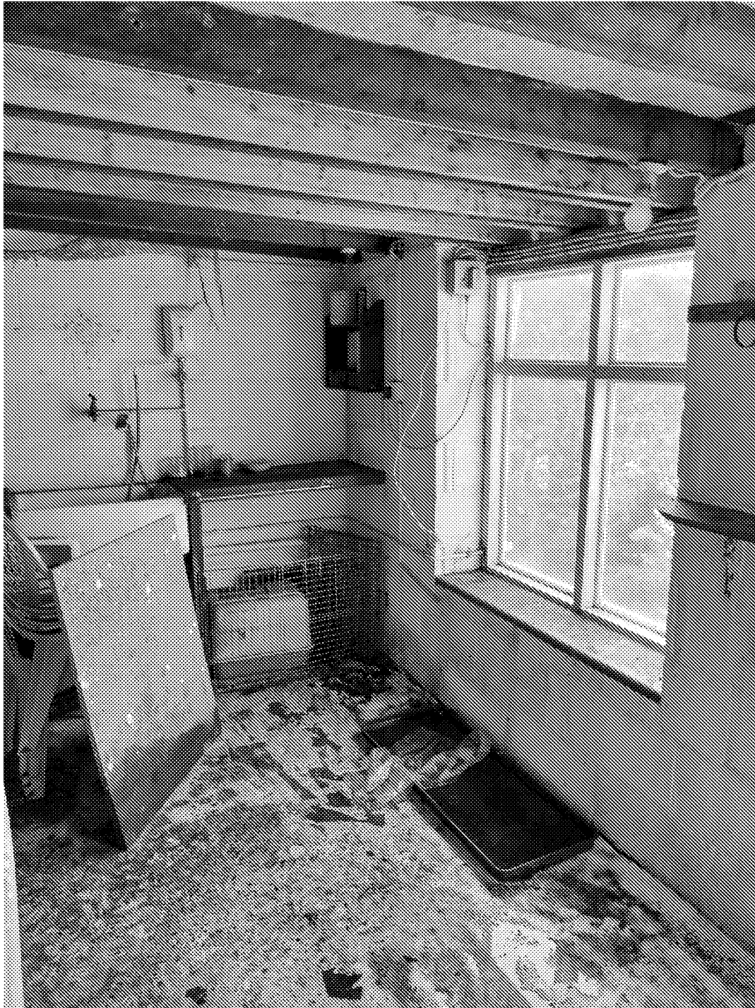
Plate VIII : Grey Barn Garage and ancillary store – Significant water ingress has lead to decay of the existing roof structure and significant issues related to dampness. Replacement of the roof will remediate these issues.
