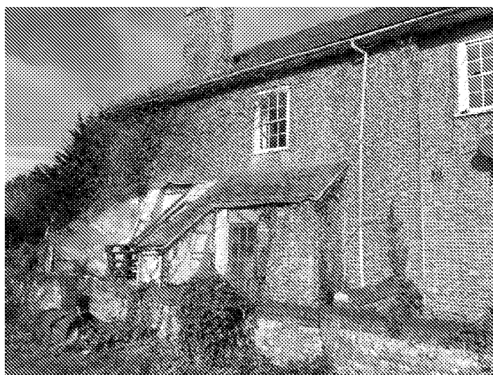
Figure 4 - The side (south) elevation with entrance porch and dilapidated conservatory
