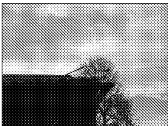
Photograph 21: Lifted lead flashing on western elevation.
