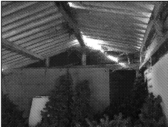
Photograph 24: Westernmost compartment of the building, showing light ingress and gaps at eaves.
