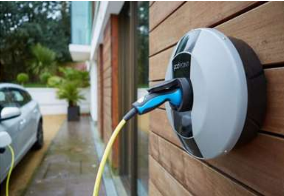
EV Charging points for all dwellings.
