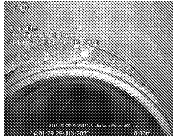
1-1-2A, 00:00:50, 0.80 m Open joint, large, PIPE HAS A TURN AT THIS POINT
