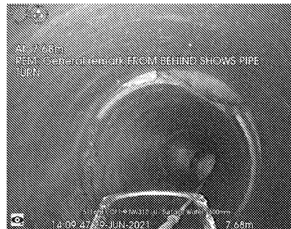
1-1-11A, 00:05:43, 7.68 m General remark, FROM BEHIND SHOWS PIPE TURN
