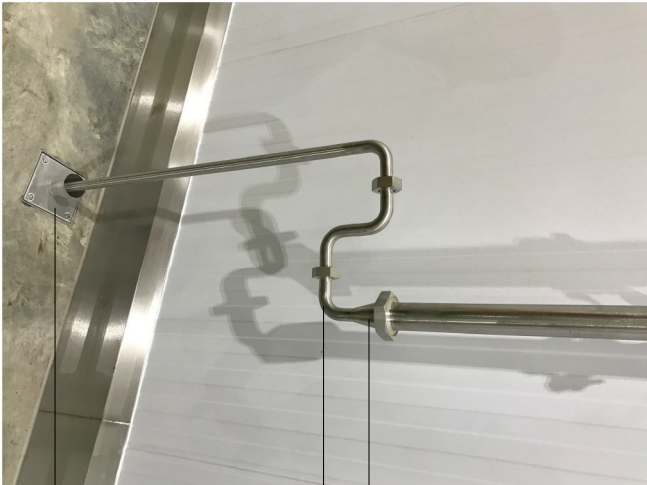
Stainless Steel Trapped Foul Gully
