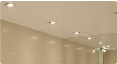
RECESSED BATHROOM DOWNLIGHTS
