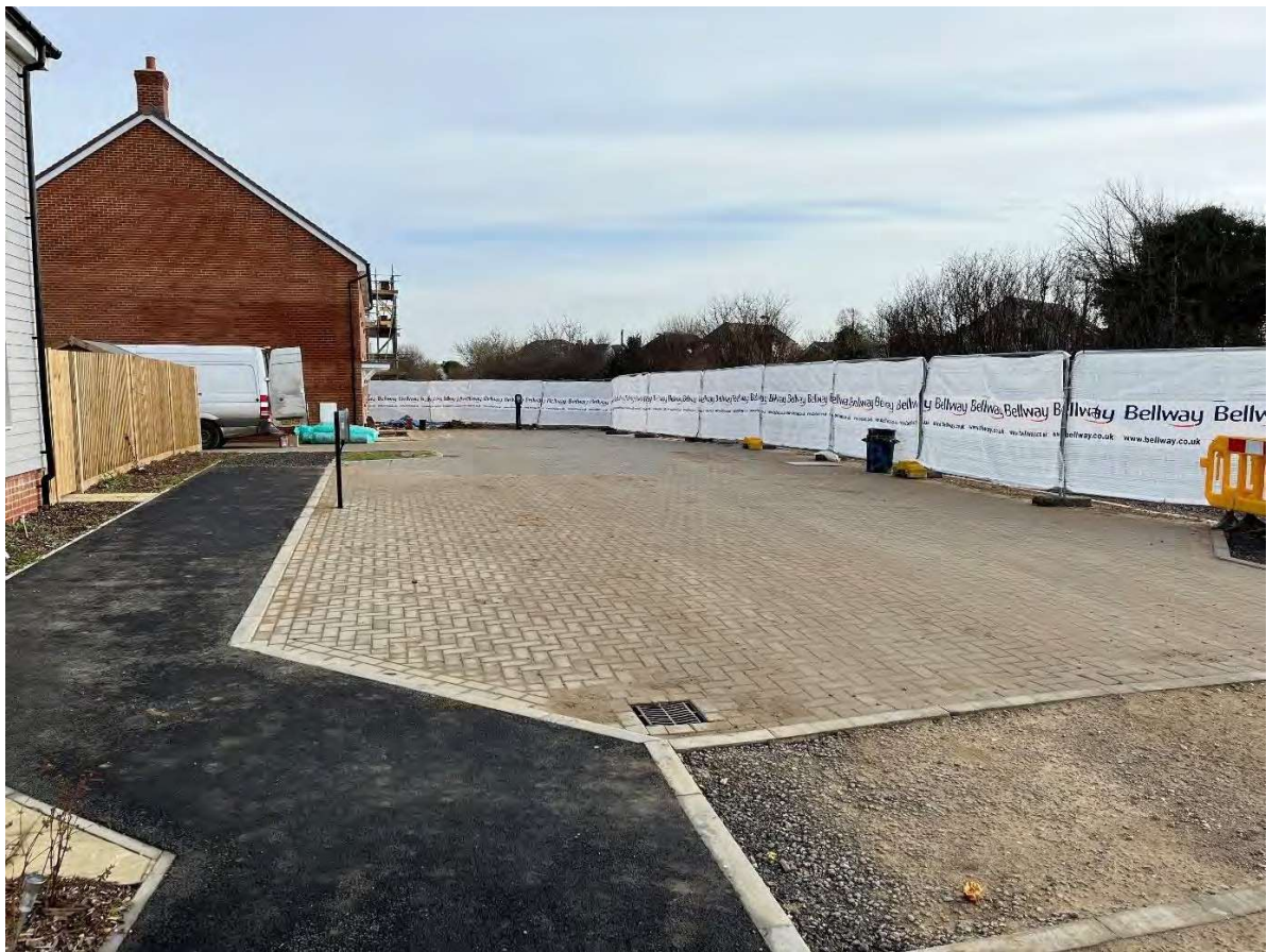
Figure 3 - Road gully in 298/300 access road
