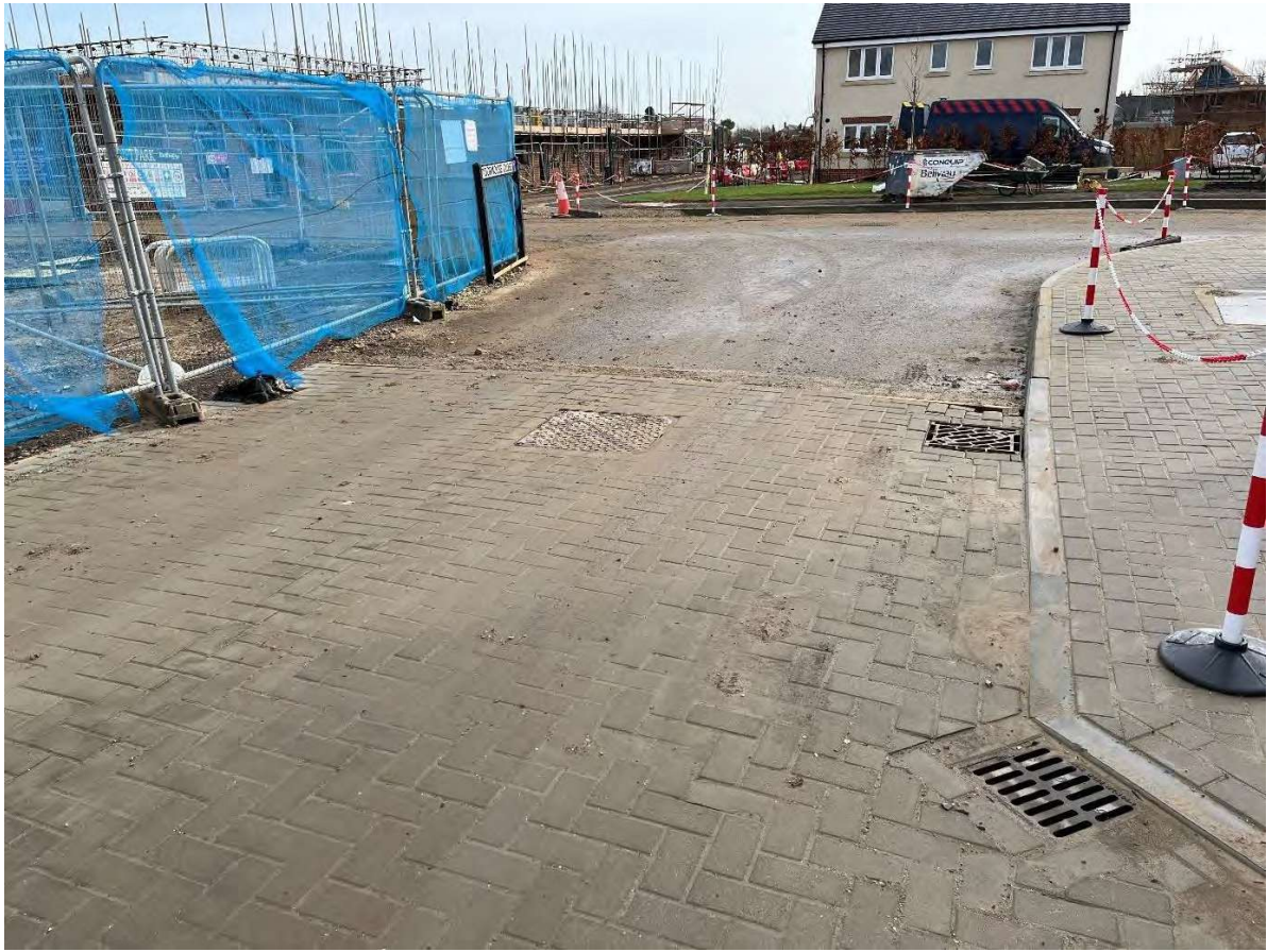
Figure 1 - Road gullies by junction adjacent to plot 9
