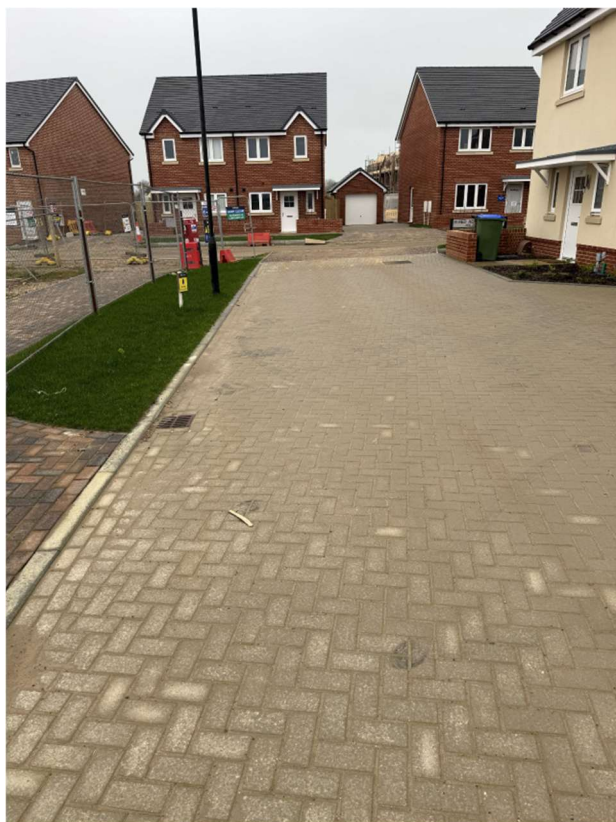
Figure 9 – Road gullies in access road to Plots 40 – 43
