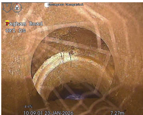
OF1X_d5858db7-6e5f-427b-ba84-24e1e03b5ca6_20260126_081105_816.jpg, 00:00:35, 7.27 m Joint displaced, large
