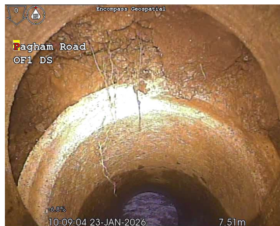
OF1X_cc650236-f2bc-46f2-88e3-bd0cc907d491_20260126_081159_363.jpg, 00:00:38, 7.51 m Finish node, other special chamber, reference: OF1 DS, FINISHES INTO THE POND OTHERSIDE OF THE DITCH
