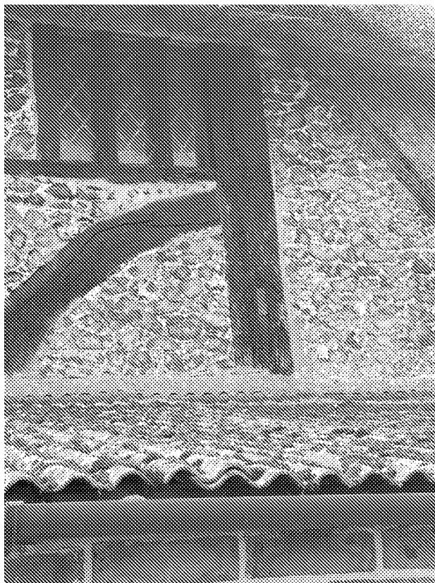
Photograph of St John's Cottage showing presence of mortice and tenon connections to existing C17 timber frame, evidencing the presence of a substantial, full width outshot.
