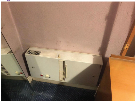
Figure 5 Ventilation Unit in Bedroom
