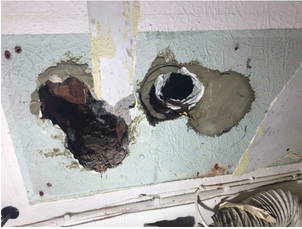
Figure 9 External wall – modern render with DPC sheet/material behind. Holes result of Ventilation units.
