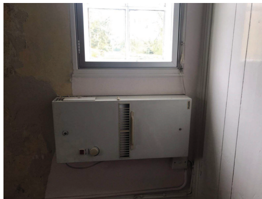
Figure 6 Ventilation unit in bedroom below window
