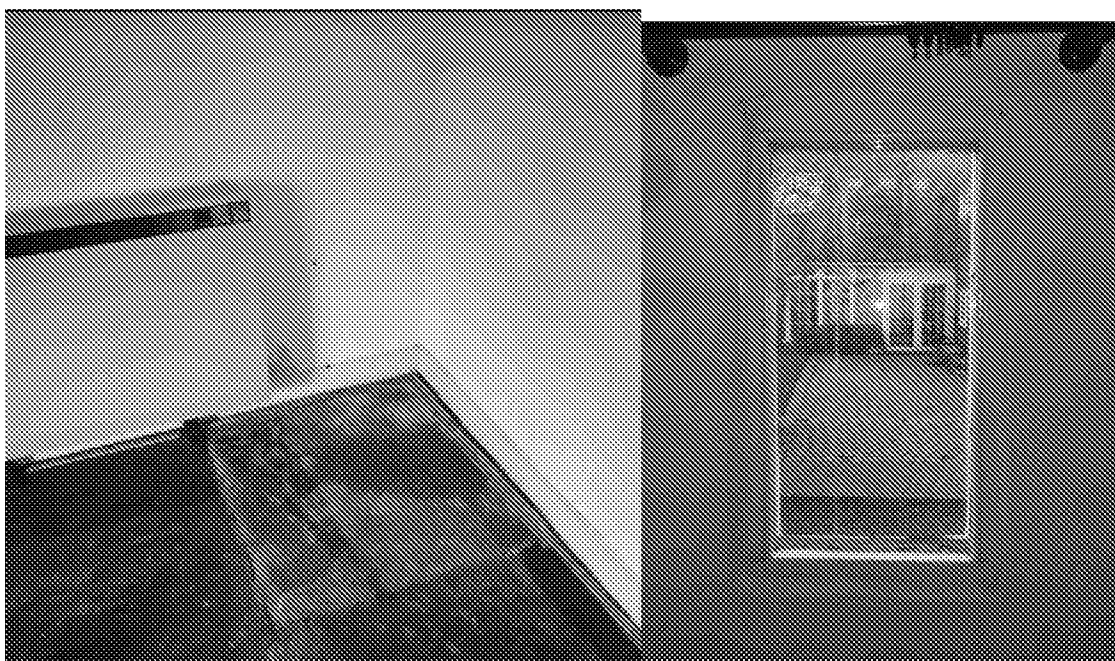
4Artex on walls and ceiling. Flaking and cracking shown near radiator
