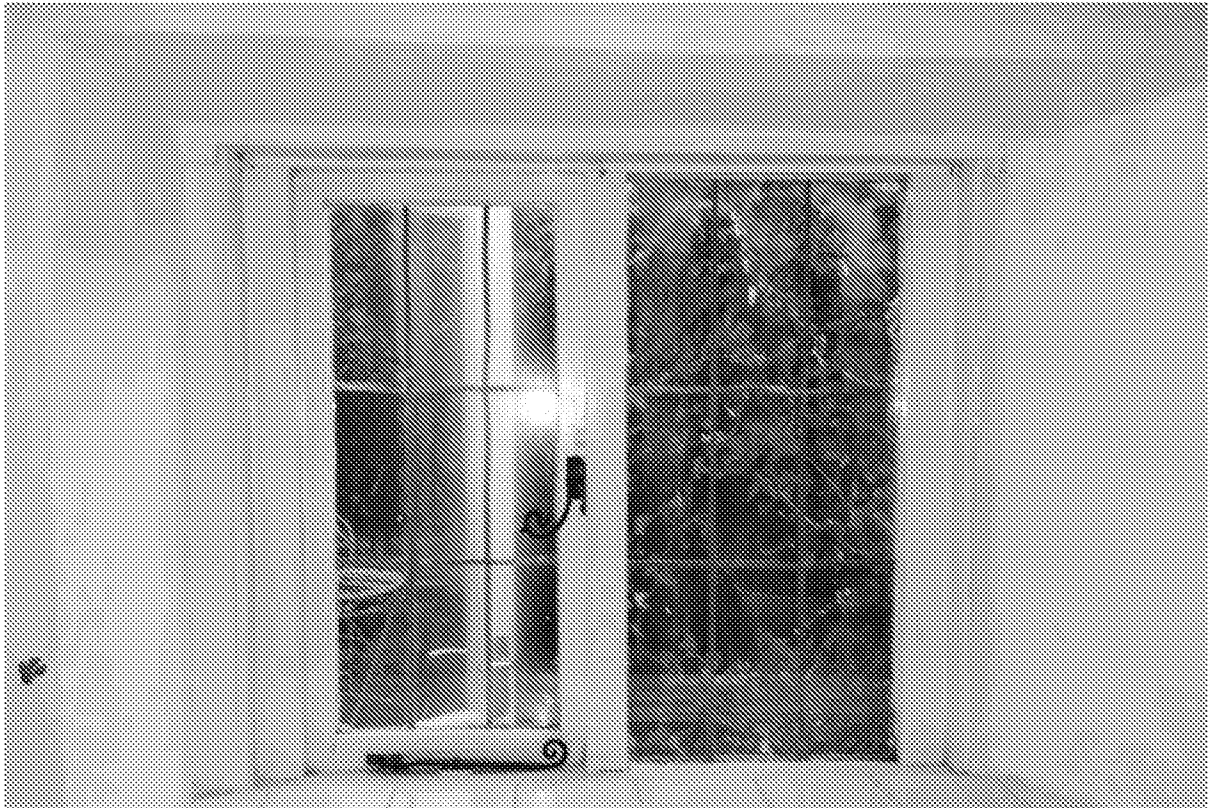
6kitchen window - sealed shut, frame beyond repair
