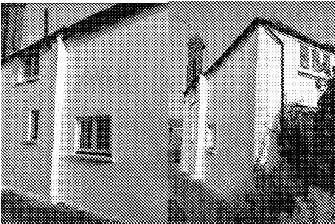
Elevations showing damp
