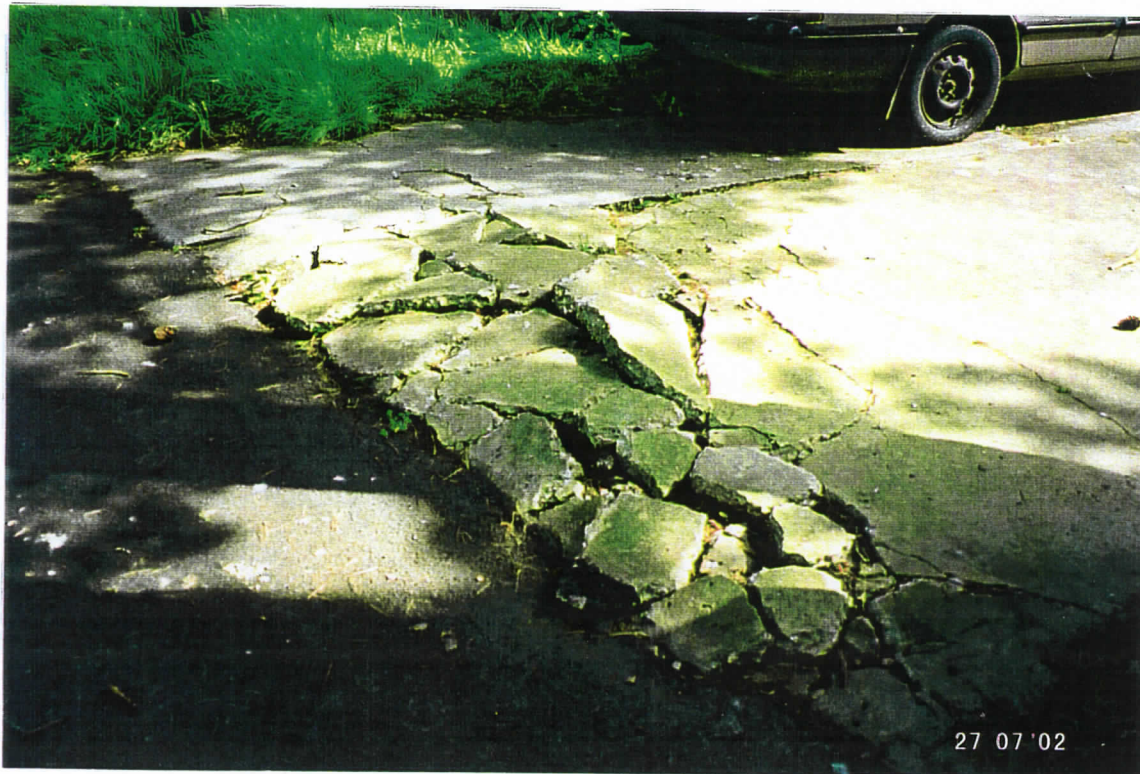
B. Area of damaged driveway.
