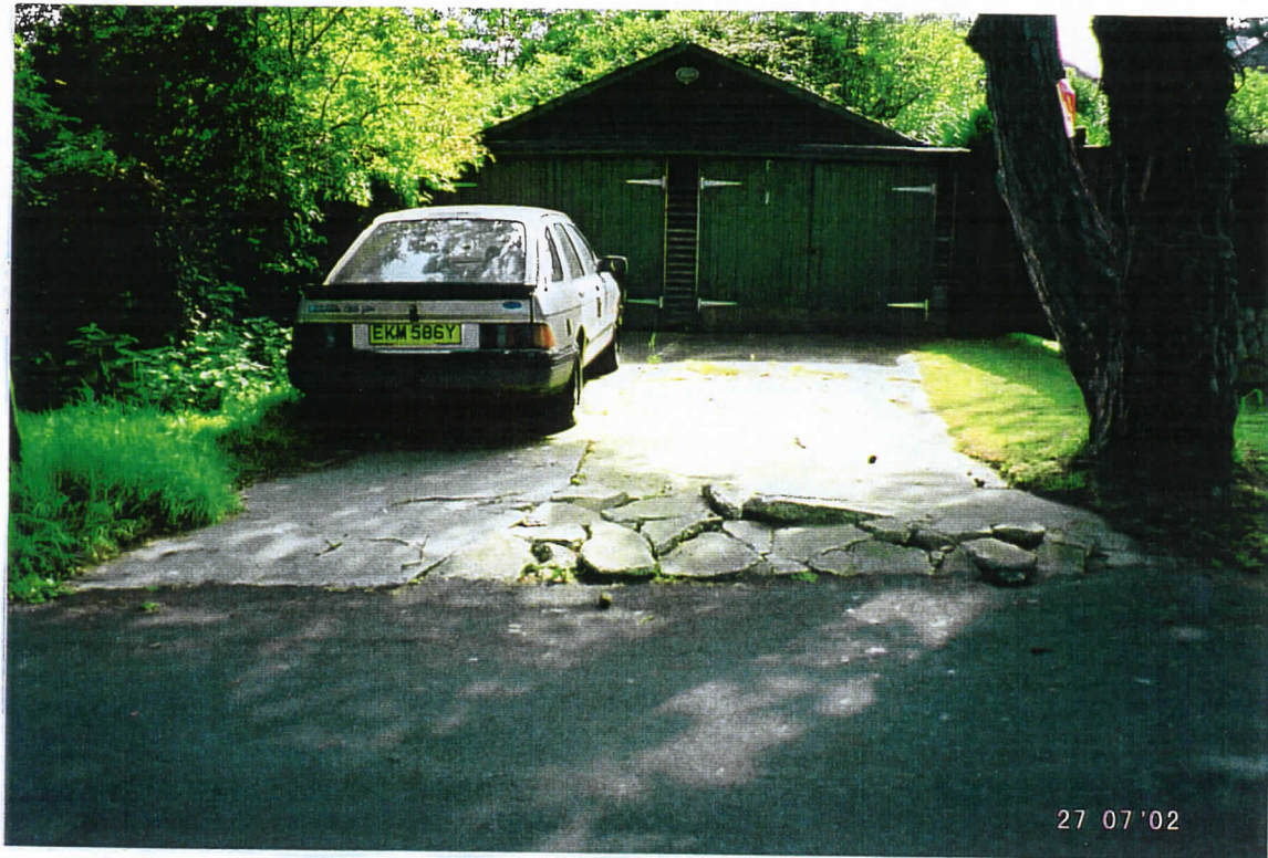
A. General view of twin drive from East Avenue. Severely damaged concrete.
