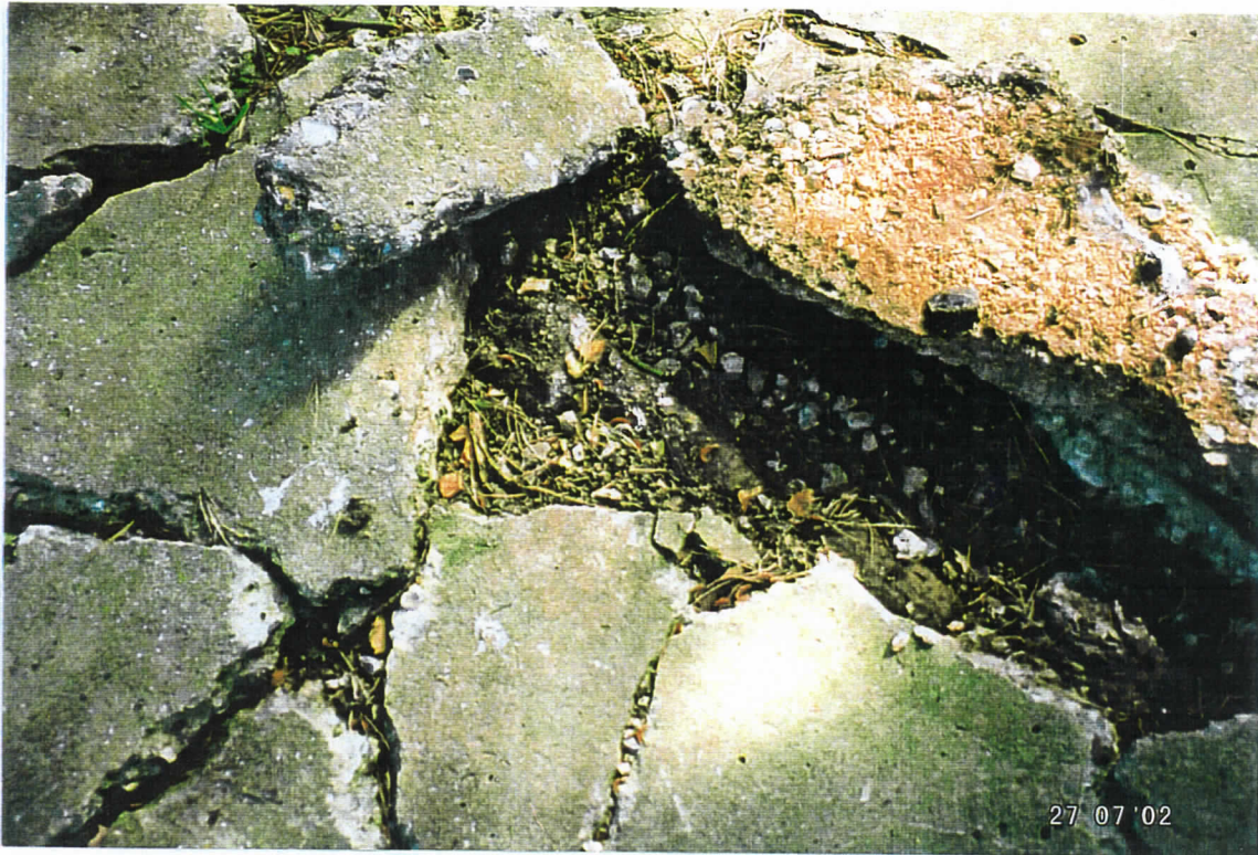
C. Root of pine tree approximately 63mm in diameter forcing up the concrete.
