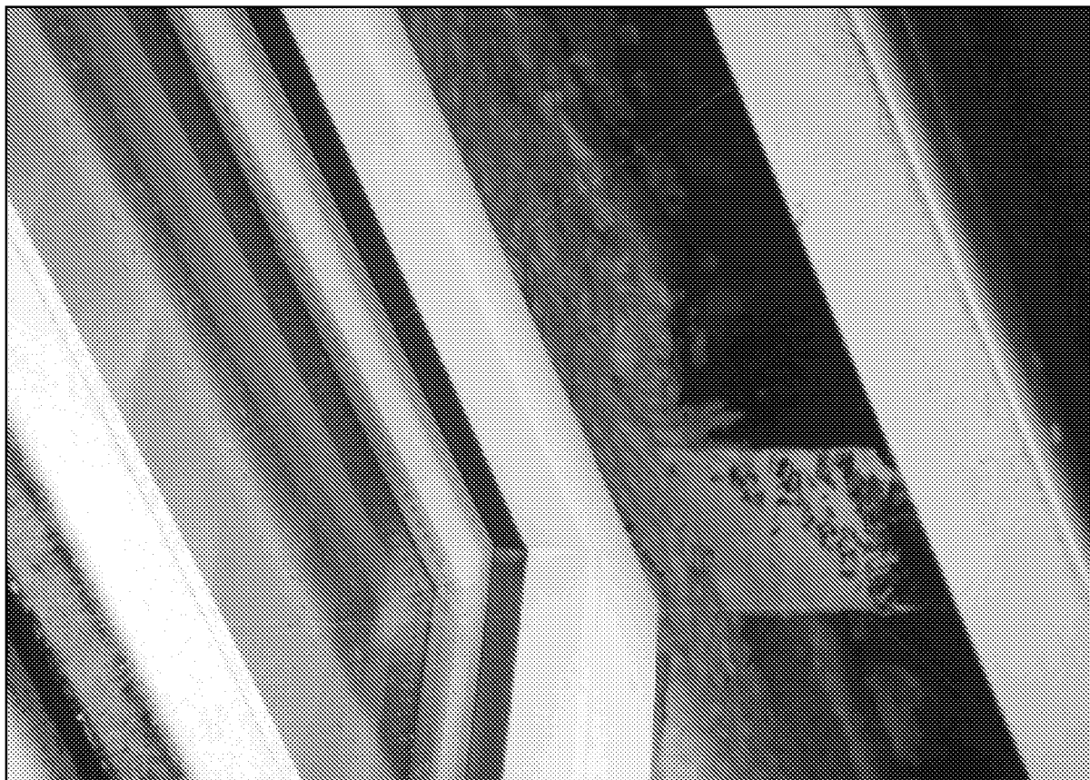
Photograph 4. Gaps between the rafters above the wall plate, under the eaves of the bungalow.
