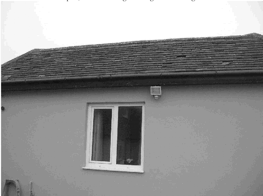
Photo 2: Missing tiles on office roof, potential access points for bats
