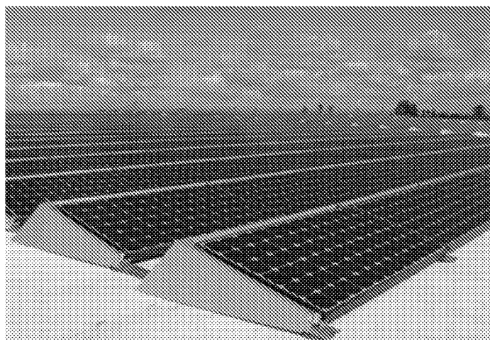
Figure 3.10: Photovoltaic array (Source: Sunpower)
