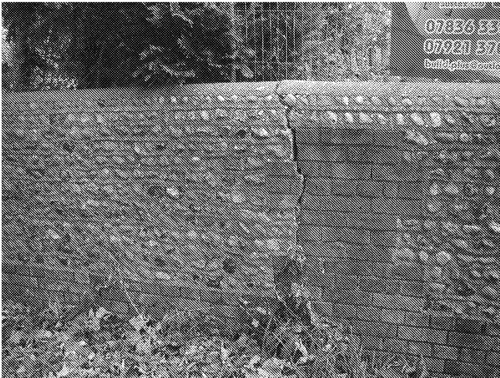
Photo – View of the existing crack in the boundary wall.
