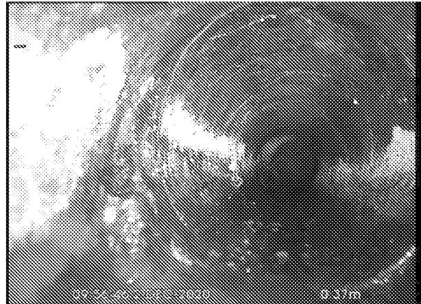
MH3X_9e5813cd-c874-42fe-90c6-71643c0676a8_20201208_215545_756.jpg, 00:00:25, 0.37 m Crack, circumferential from 12 o'clock to 12 o'clock
