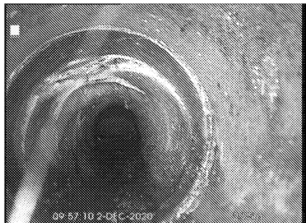
MH3X_9e064088-caa3-4ea0-819c-19b170f6255e_20201208_215628_379.jpg, 00:00:48, 2.75 m Hole in drain or sewer from 9 o'clock to 12 o'clock
