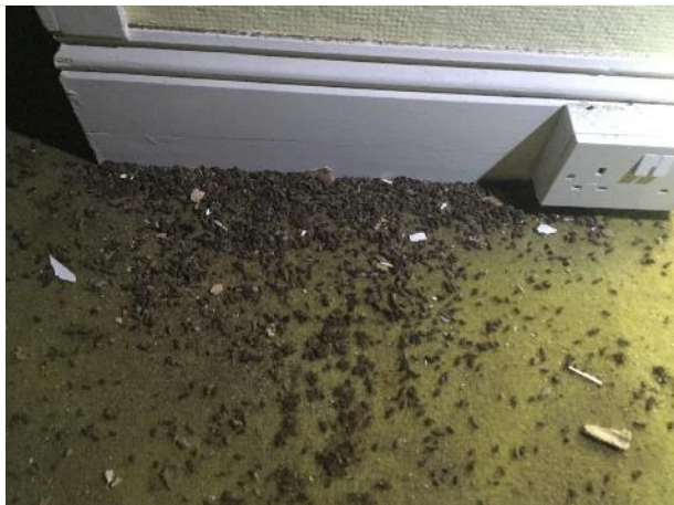
Serotine bat droppings present in the main house.
