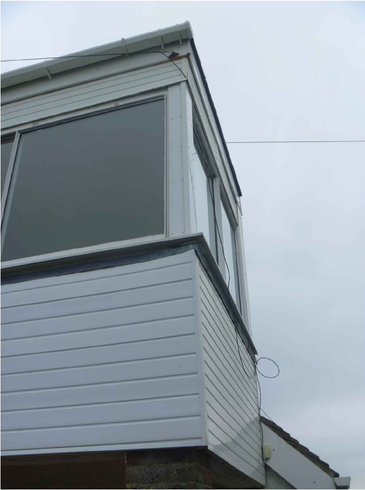
+PH UPVC windows and cladding - out of character with the host building
