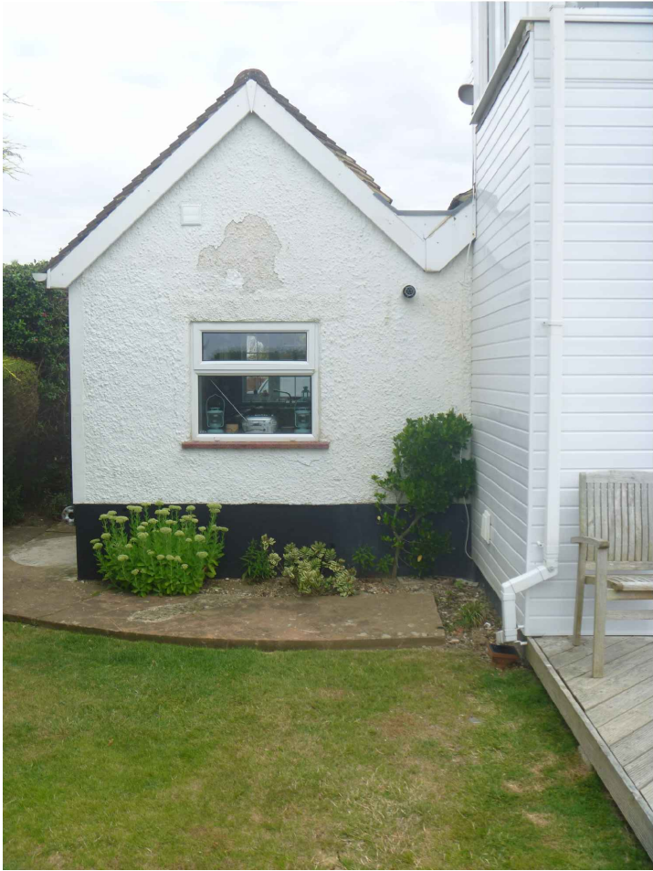
+PH Failing render on south elevation
