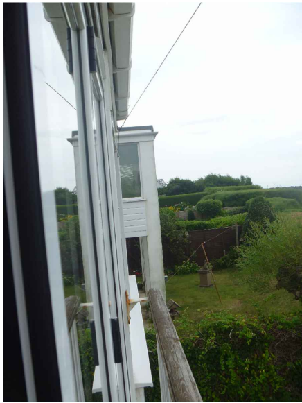
+PH Neighbours extension protruding over building line
