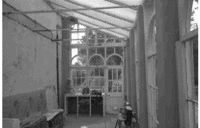
Internal View of Conservatory – Please observe non original UPVC glazing to roof structure.
