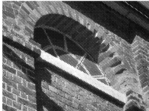
Fig 5. Damaged brickwork over platform.
