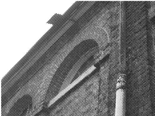
Fig 4. Loose roof tiling over platform
