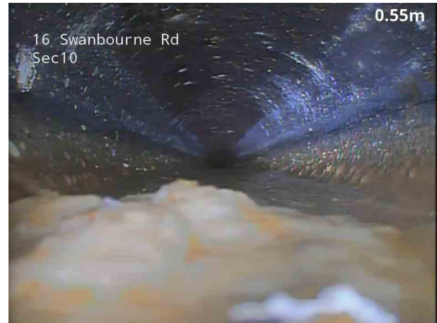
2, 00:00:07, 0.50 m Attached deposits, fouling from 5 o'clock to 7 o'clock, 10% cross-sectional area loss
