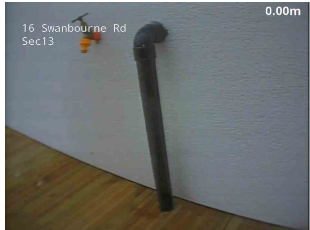
2, 00:00:12, 0.00 m Finish node, manhole, reference: FP, Suspected concealed FWG
