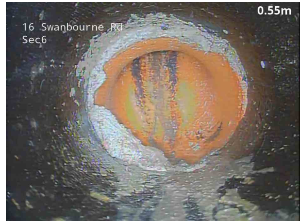
2, 00:00:18, 0.80 m Attached deposits, other at joint from 6 o'clock to 9 o'clock, 5% cross-sectional area loss, Jointing compound
