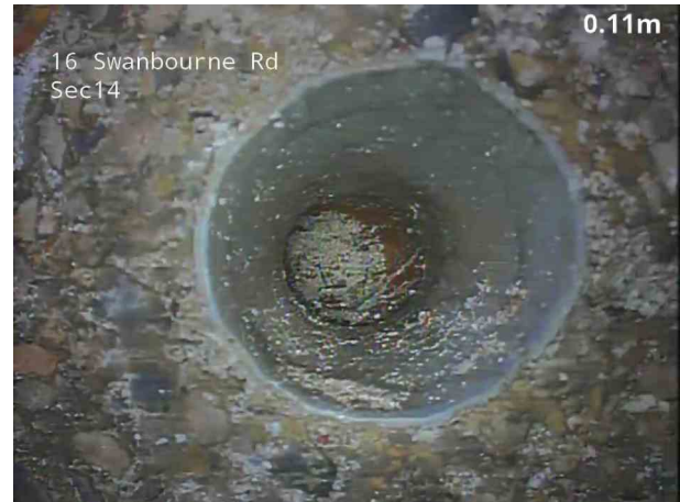
2, 00:00:08, 0.00 m Survey abandoned, Unable to survey, assumed to discharge to soakaway
