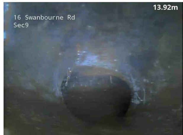
6, 00:01:05, 14.00 m Line deviates down
