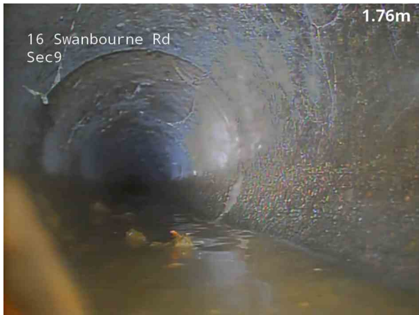
3, 00:00:15, 1.80 m Attached deposits, fouling from 4 o'clock to 8 o'clock, 10% cross-sectional area loss, change
