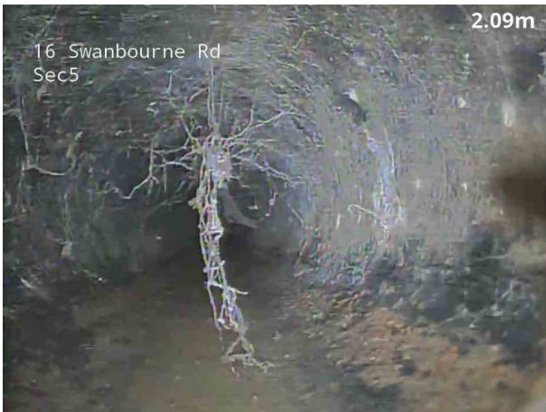
3, 00:00:41, 2.10 m Settled deposits, fine, 5% cross-sectional area loss, finish
