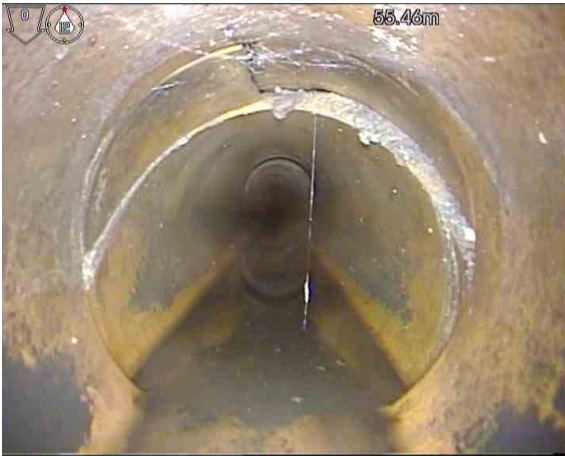
1, 00:04:22, 55.46 m Broken pipe from 9 o'clock to 3 o'clock
