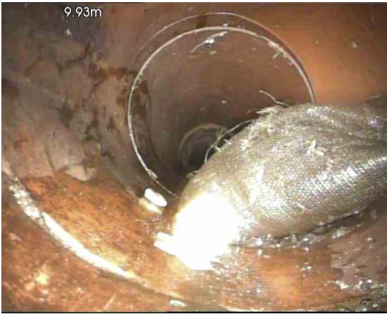
1, 00:01:21, 10.44 m Defective junction, blocked at 3 o'clock, diameter: 150mm
