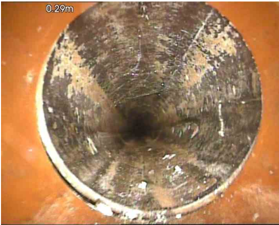
1, 00:00:10, 0.29 m Joint displaced, medium
