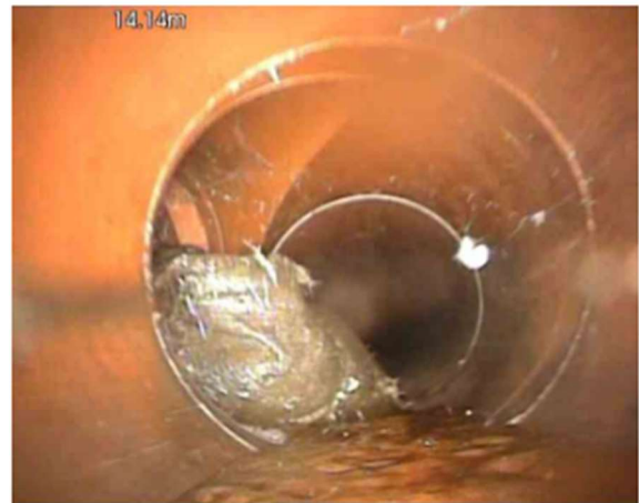
1, 00:00:35, 14.14 m Defective junction, blocked at 9 o'clock, diameter: 150mm
