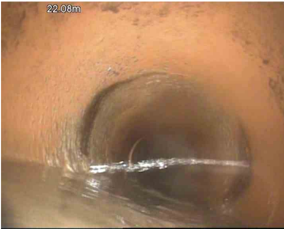
1, 00:01:26, 22.24 m Infiltration, running at joint at 3 o'clock
