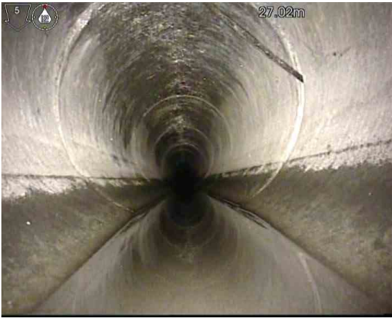
1, 00:02:12, 27.64 m Sealing ring intruding, hanging above centre from 10 o'clock to 4 o'clock, 27.02
