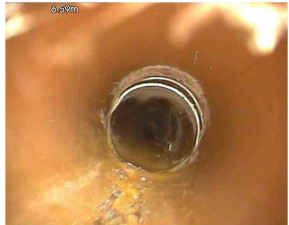
1, 00:00:24, 6.59 m Joint displaced, medium
