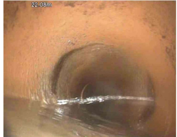
1, 00:01:26, 22.24 m Infiltration, running at joint at 3 o'clock
