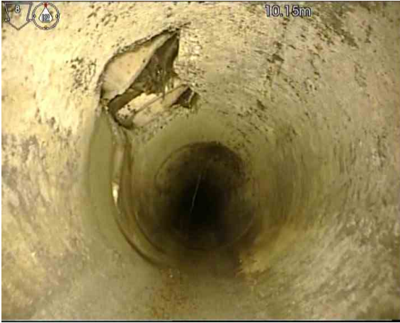
1, 00:00:52, 10.22 m Connection defective, connecting pipe is damaged at 10 o'clock, diameter: 150mm
