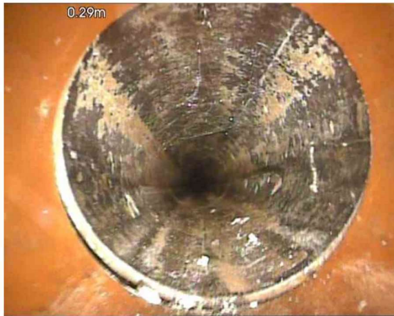
1, 00:00:10, 0.29 m Joint displaced, medium
