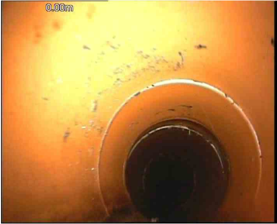
1, 00:00:08, 0.20 m Joint displaced, medium
