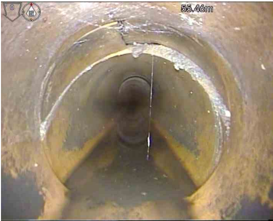
1, 00:04:22, 55.46 m Broken pipe from 9 o'clock to 3 o'clock
