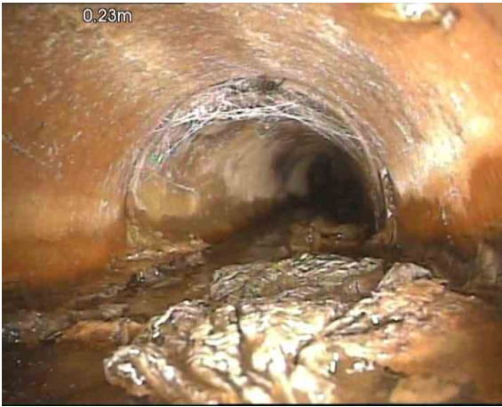
1, 00:00:11, 0.23 m Settled deposits, hard or compacted, 20% cross-sectional area loss
