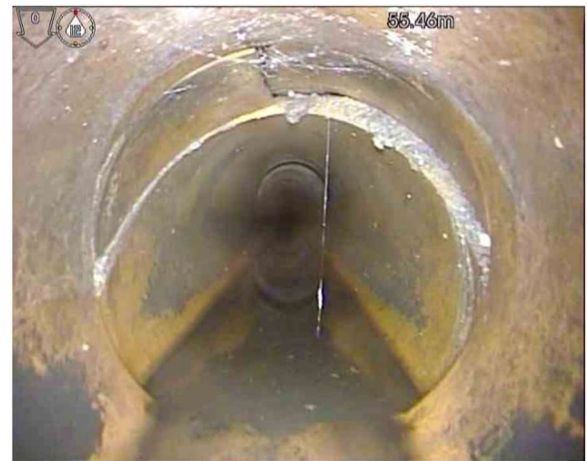
1, 00:04:22, 55.46 m Broken pipe from 9 o'clock to 3 o'clock
