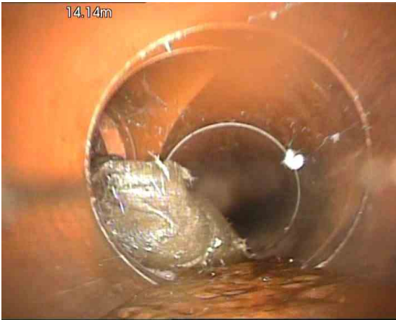
1, 00:00:35, 14.14 m Defective junction, blocked at 9 o'clock, diameter: 150mm
