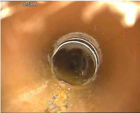
1, 00:00:24, 6.59 m Joint displaced, medium
