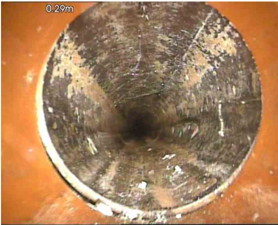
1, 00:00:10, 0.29 m Joint displaced, medium
