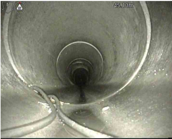
1, 00:03:04, 45.13 m Sealing ring intruding, intruding but not hanging from 3 o'clock to 9 o'clock
