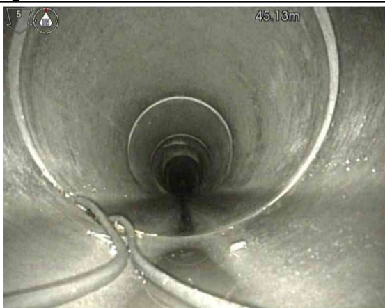
1, 00:03:04, 45.13 m Sealing ring intruding, intruding but not hanging from 3 o'clock to 9 o'clock
