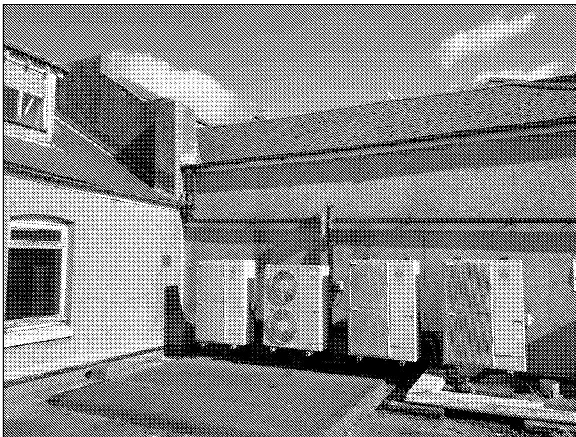
Existing AC units
