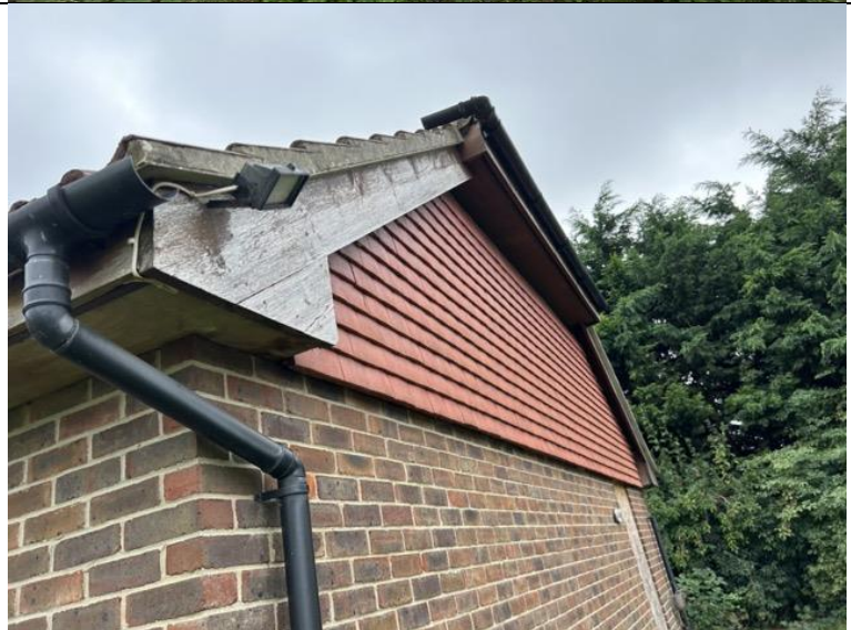
Photograph 14: Building 1. Hanging tiles can be seen.
