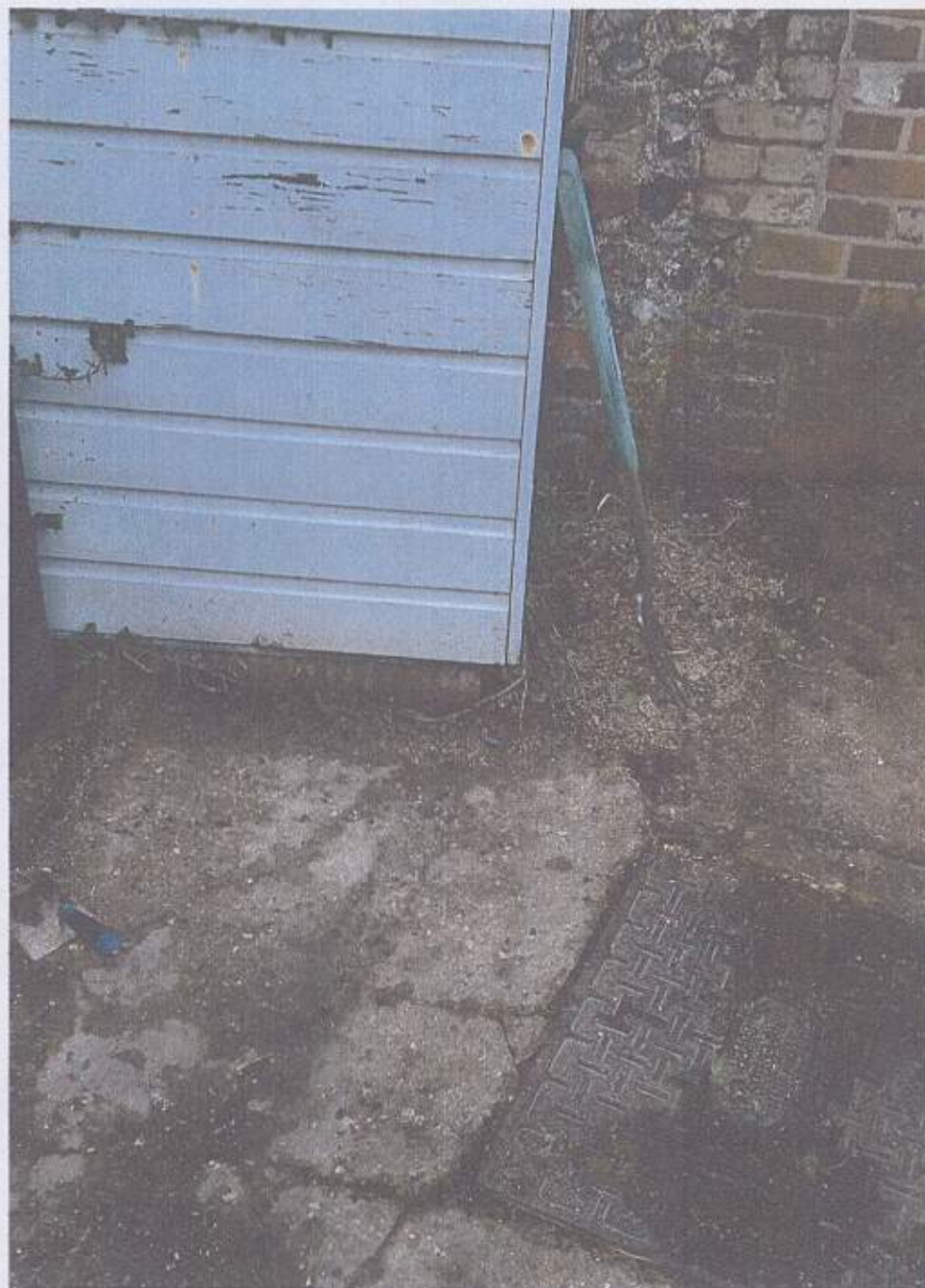
NON ORIGINAL PLASTIC CLAD LINK - LOWER LEVEL - TO BE DEMOLISHED
