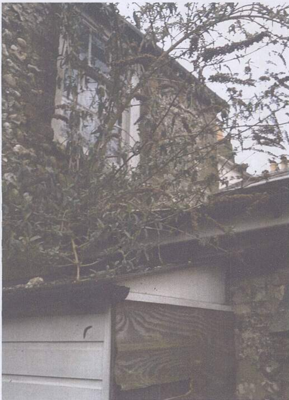
NON ORIGINAL PLASTIC CLAD LINK - UPPER LEVEL - TO BE DEMOLISHED
