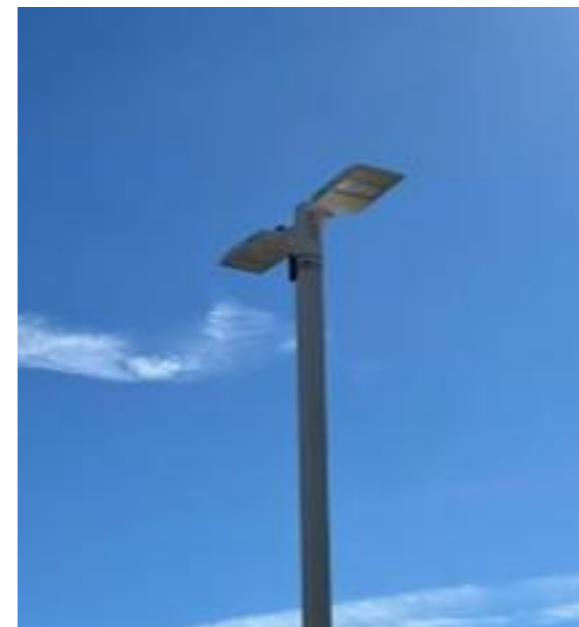
Pole Mounted Lighting
