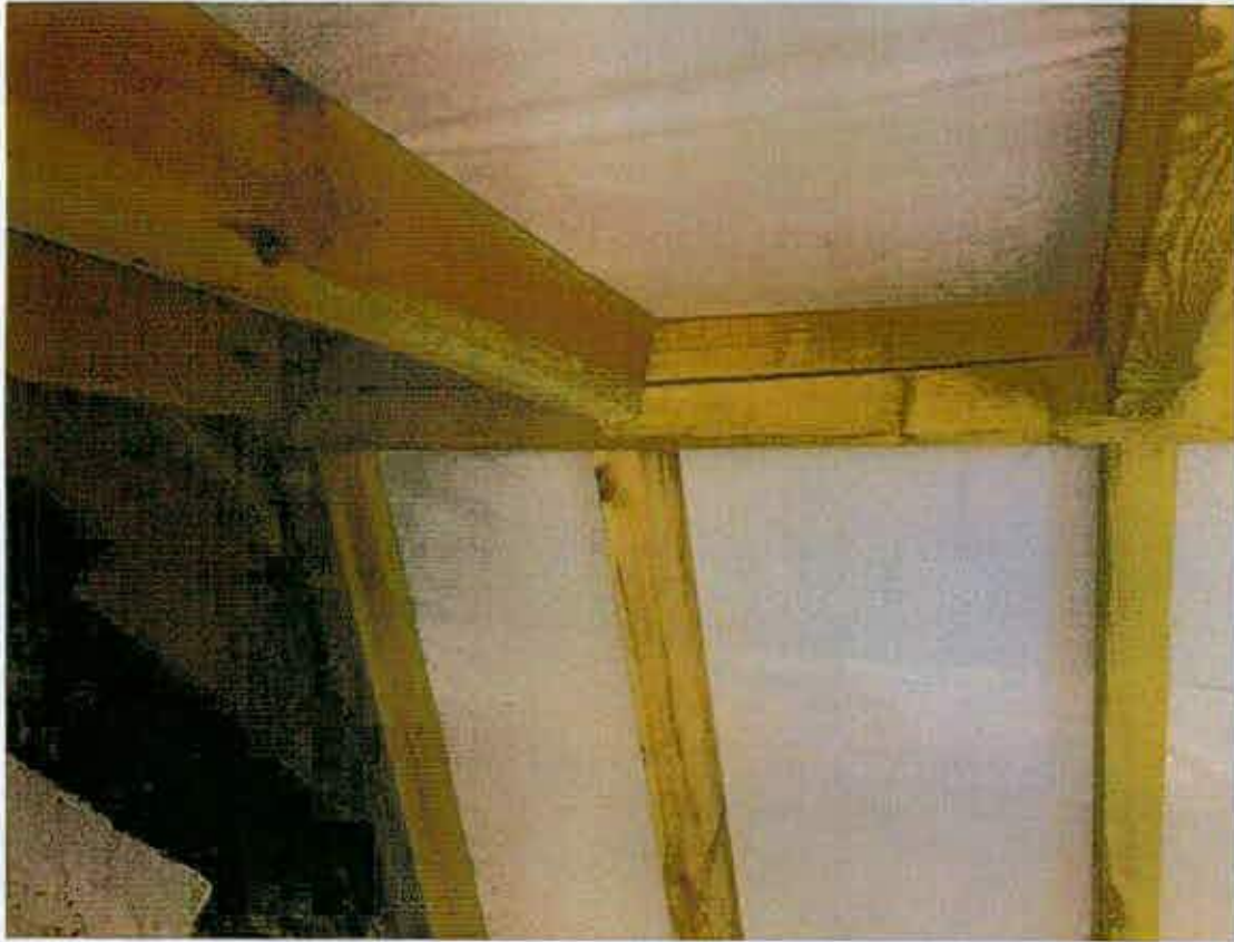
Internal view of roof structure. Main beam cracking and causing sagging.
