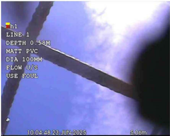
L1X_b208af46-6f25-4ce0-b5a9-73d6107d076e_20250701_165639_272.jpg, 00:00:28, 5.06 m Finish node, other special chamber, reference: L1
