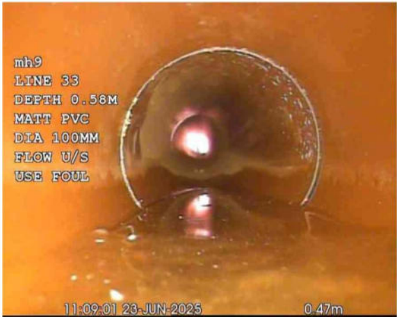
L33X_21a7342b-2438-4a3f-a4d1-a4bb3c42f243_20250701_1 70813_347.jpg, 00:00:06, 0.47 m Water level, 5% of the vertical dimension
