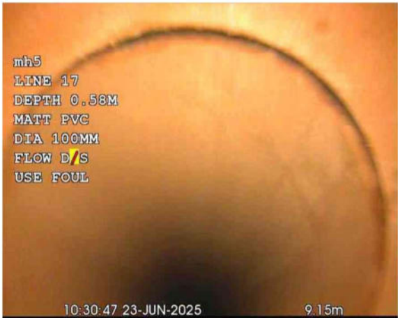
MH 5X_84b027ab-51f7-4928-a7e0-1d0c026f51b7_20250701_1700 035_892.jpg, 00:00:30, 9.15 m Line deviates down
