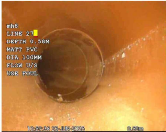
L27X_ddb0d084-8b81-450a-921b-cdab44ff2023_20250701_170657_353.jpg, 00:00:05, 0.50 m Line deviates left
