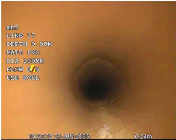
MH 5X_79554204-539b-43bf-9e42-5e1eb01cfb4e_20250701_1700 034_661.jpg, 00:00:05, 0.24 m Pipe material changes to vitrified clay at this point
