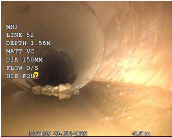
MH 3X_cd882e98-e9b0-49f6-88cb-8ad3bf3c588e_20250701_171 346_507.jpg, 00:00:00, 0.00 m Start node, manhole, reference: FMH52
