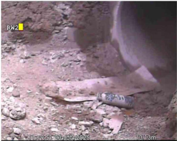
RW1X_25a4fa14-6ce2-47e6-be28-dda2abd915fd_20250701_170838_272.jpg, 00:01:01, 13.13 m Finish node, manhole, reference: SMH32
