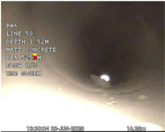
RW 6X_3b52f4c5-18b4-459b-8301-7d3856c56ca3_20250701_171 259_239.jpg, 00:01:17, 16.25 m Connection other than junction at 2 o'clock, 150mm dia
