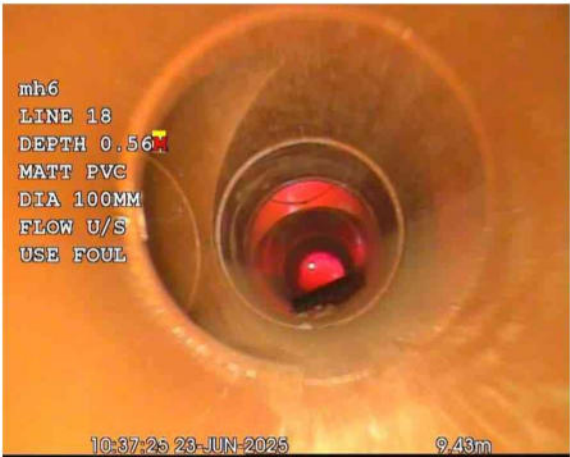
L18X_95c00c07-51e8-4ff7-afce-76ff066155ea_20250701_170048_363.jpg, 00:00:31, 9.43 m Junction at 9 o'clock, 100mm dia
