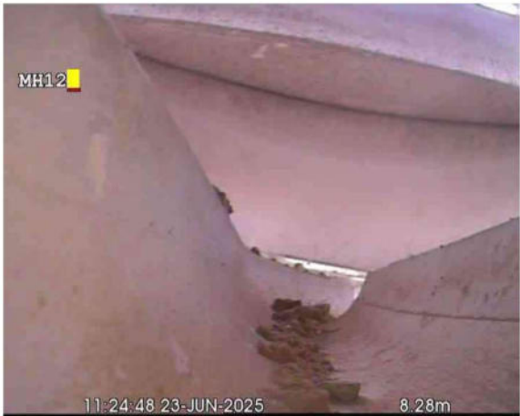
MH 11X_52ea81d8-a3e5-4f90-a435-5e0d3a37668b_20250701_1 70909_809.jpg, 00:00:29, 8.28 m Finish node, manhole, reference: FMH77
