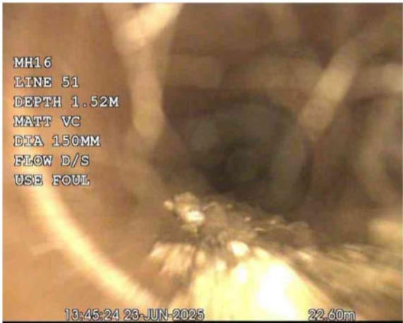
MH 16X_49207387-fce9-4f86-a358-b32d11aac392_20250701_17 1322_631.jpg, 00:00:44, 22.60 m Junction at 2 o'clock, 150mm dia
