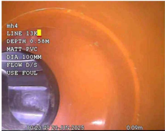
MH 4X_975fb1c5-2f44-413c-a3e1-faeccf9ba1cf_20250701_16593 1_628.jpg, 00:00:04, 0.09 m Line deviates left
