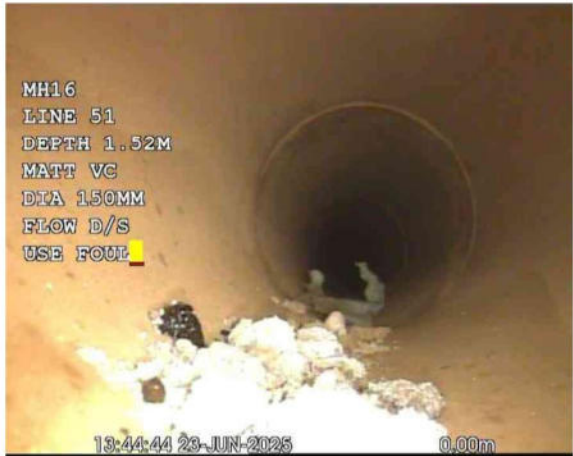
MH 16X_831be70e-b5d3-4fd3-a591-6508bf28d573_20250701_17 1316_109.jpg, 00:00:03, 0.00 m Settled deposits, coarse, 10% cross-sectional area loss
