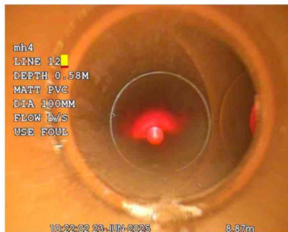
L12X_5ce7d6ae-ff7a-4a0d-b4d9-cc27464934ca_20250701_165921_952.jpg, 00:00:34, 8.87 m Junction at 3 o'clock, 100mm dia
