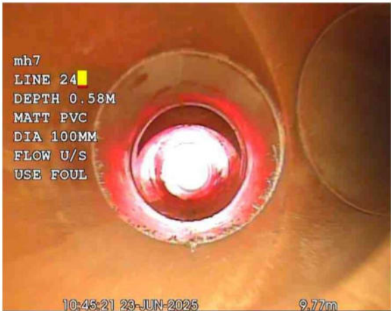
L24X_edb9189f-978a-4e52-a46c-f695935820cc_20250701_170241_508.jpg, 00:00:27, 9.77 m Junction at 3 o'clock, 100mm dia
