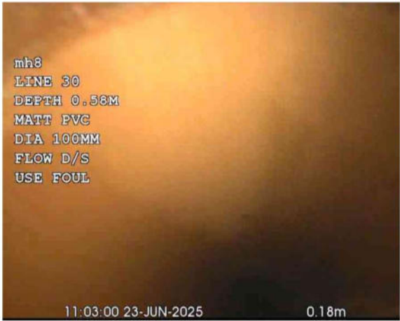
MH 8X_6e208c22-d6a4-4988-92a0-0fb0cd3422ce_20250701_170 728_259.jpg, 00:00:04, 0.18 m Pipe material changes to vitrified clay at this point
