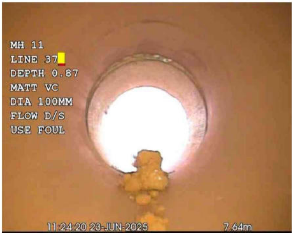
MH 11X_91691825-464d-4d15-ba6c-5119b173f1fa_20250701_17 0908_566.jpg, 00:00:25, 7.64 m Settled deposits, coarse, 15% cross-sectional area loss
