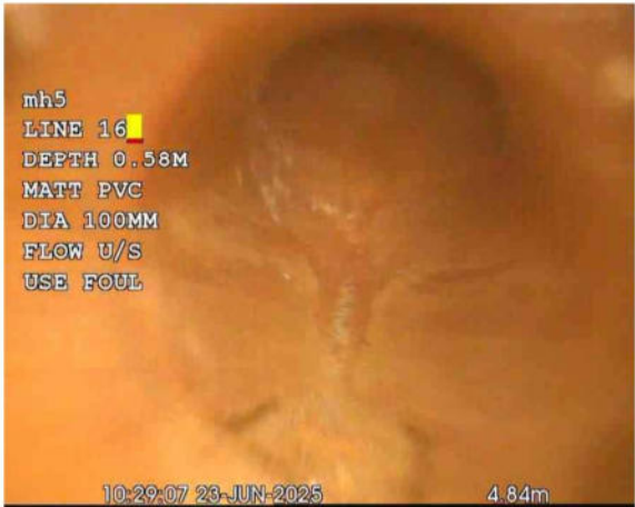
L16X_2b70c7af-9f89-49f3-9f3e-118ce13f01d9_20250701_170017_910.jpg, 00:00:19, 4.84 m Line deviates up
