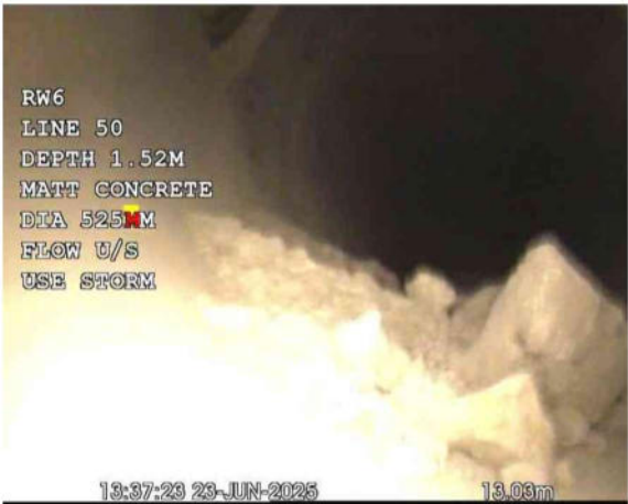
RW 6X_41c2864b-3924-4bc4-96b7-07289dc46039_20250701_17 1257_433.jpg, 00:00:35, 13.03 m Settled deposits, coarse, 10% cross-sectional area loss
