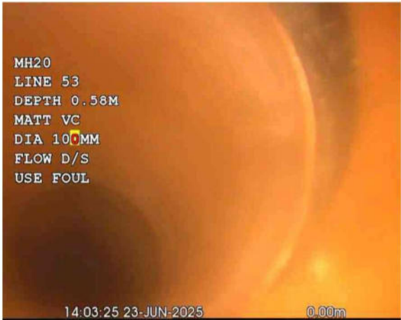
MH 20X_46c1ffb-e7ae8-44dc-b555-49cfe8c7dc1c_20250701_164 240_563.jpg, 00:00:00, 0.00 m Start node, manhole, reference: FIC16
