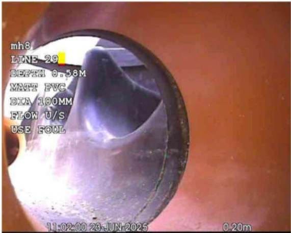
MH 9X_ff6d5cc7-60f5-4b17-87d1-b45710adc309_20250701_1707 22_563.jpg, 00:00:04, 0.20 m Line deviates left
