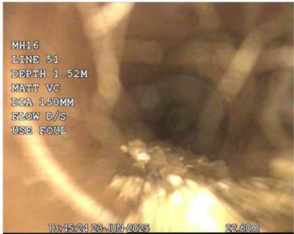
MH 16X_ae6637d3-2ee9-4e78-8611-e4a6e2d9159e_20250701_1 71324_926.jpg, 00:00:44, 22.60 m Settled deposits, coarse, 10% cross-sectional area loss
