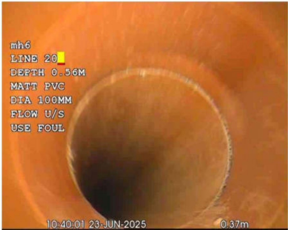
L20X_e231ad4f-6329-4834-bbd9-60ce2bfd9fef_20250701_17 0138_447.jpg, 00:00:06, 0.37 m Line deviates left
