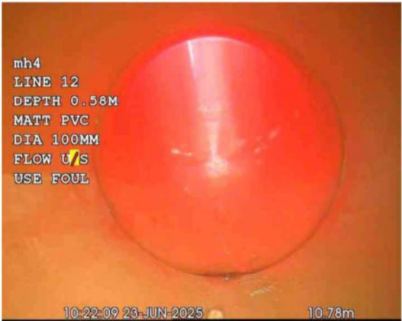
L12X_8838090a-ad35-4fa0-95ed-027d46885759_20250701_165924_960.jpg, 00:00:41, 10.78 m Line deviates up
