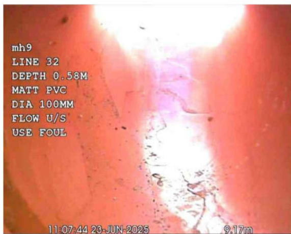
L32X_15bb80fe-d993-43e1-b97b-02fa2b90178f_20250701_1 70804_974.jpg, 00:00:36, 9.17 m Line deviates up
