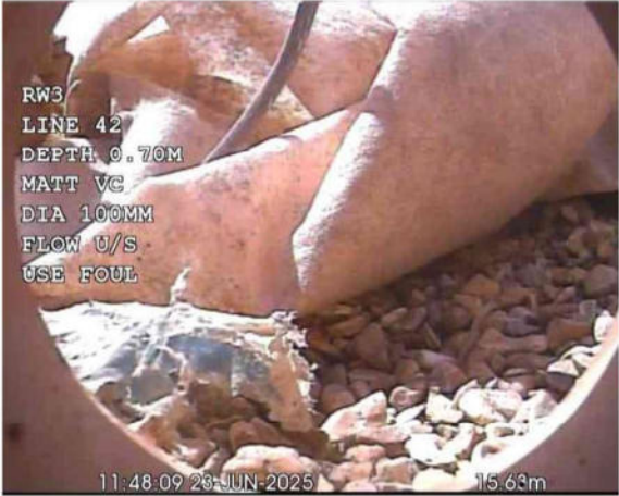
L42X_671d8aa7-91ea-4559-851a-df5ee5461d31_20250701_171105_580.jpg, 00:00:51, 15.63 m Finish node, other special chamber, reference: PPCP4
