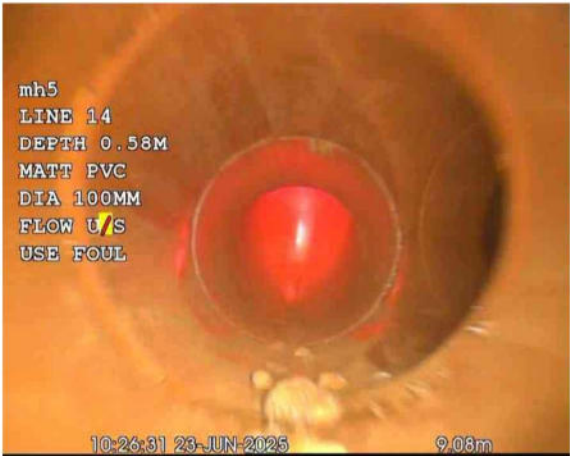
L14X_48e92ebe-8d23-4adb-b3a8-6b40c62f347c_20250701_165946_565.jpg, 00:00:28, 8.90 m Junction at 3 o'clock, 100mm dia
