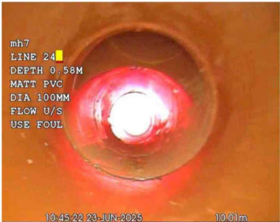
L24X_95e10676-0d75-4700-ac2f-92c8a77e2404_20250701_170242_738.jpg, 00:00:27, 10.01 m Junction at 12 o'clock, 100mm dia
