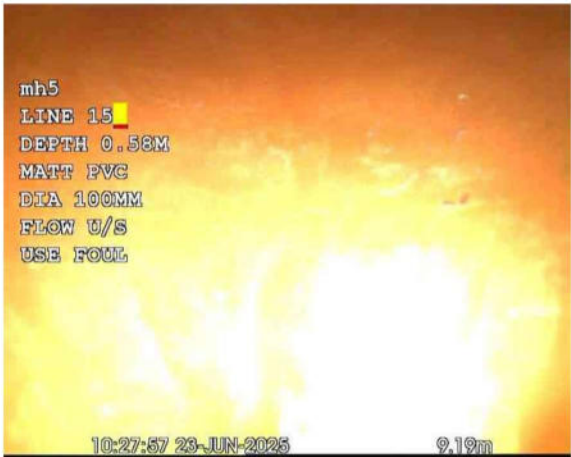
L15X_314e08ad-9e8b-4d72-8cff-b7717ed69cd0_20250701_170007_949.jpg, 00:00:33, 9.19 m Line deviates up
