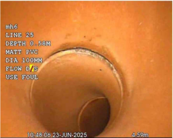
MH 6X_dd7489f3-b8fd-4936-8070-ffeff079b4e4_20250701_17025 6_010.jpg, 00:00:24, 4.59 m Line deviates down
