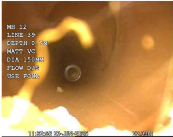
MH 12X_ae8ecd57-5ba5-4875-9bd5-2c010693ccb7_20250701_170942_601.jpg, 00:00:53, 22.23 m Junction at 2 o'clock, 150mm dia
