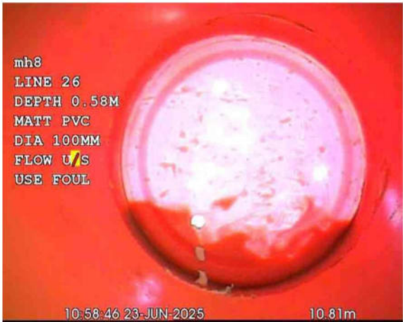
L26X_d77d8a73-98da-43ca-9dc7-078ef4fa5d41_20250701_170335_231.jpg, 00:00:38, 10.81 m Finish node, other special chamber, reference: L26
