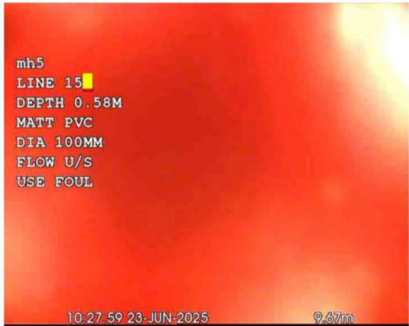
L15X_e8db75b0-d803-4588-9c0a-4334eb6471ef_20250701_170009_182.jpg, 00:00:36, 9.76 m Finish node, other special chamber, reference: L15
