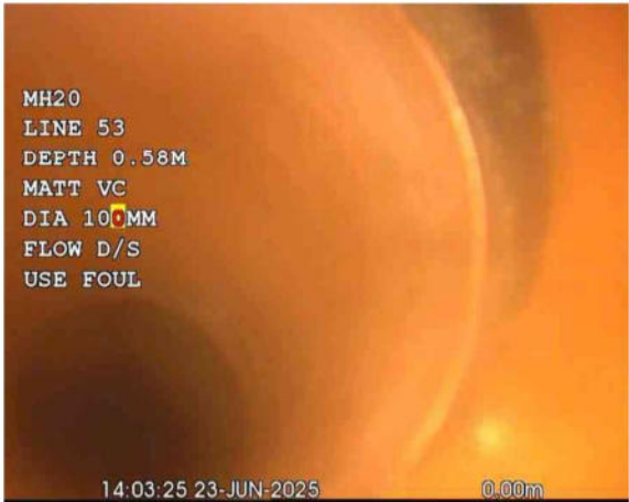
MH 20X_19a75c38-5faa-45f8-801b-16fc79676ae1_20250701_171 404_367.jpg, 00:00:01, 0.00 m Line deviates down
