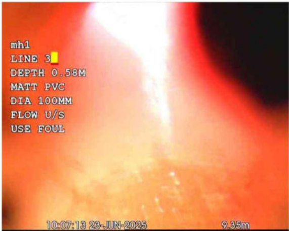
L3X_a26419ca-6fb5-48c6-ab7a-cec7713e4c82_20250701_165704_269.jpg, 00:00:22, 9.35 m Line deviates up
