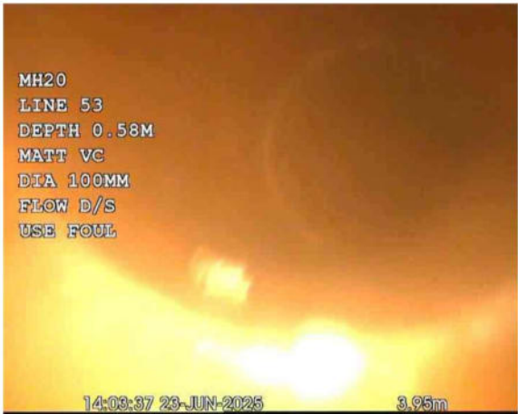
MH 20X_64f35a48-bdcb-4e49-97a6-66b6e013821a_20250701_17 1406_201.jpg, 00:00:13, 3.95 m Line deviates right
