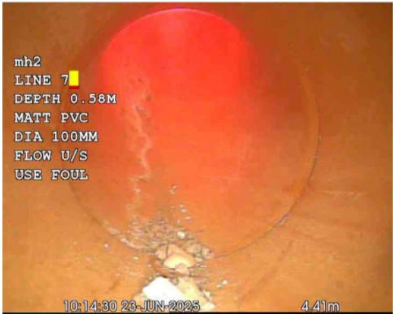
L7X_d8a5b776-61d9-4dee-b049-ee94d4a66250_20250701_1 65808_887.jpg, 00:00:22, 4.41 m Line deviates up
