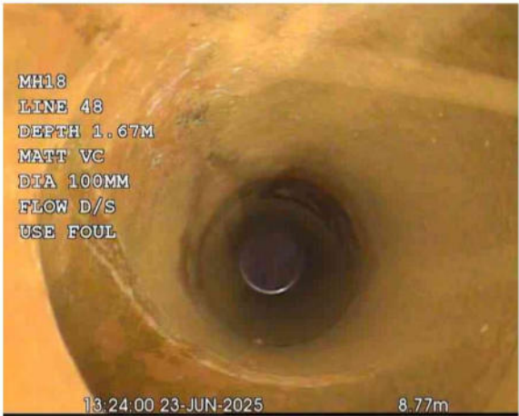
MH 18X_90cf7bcf-f849-4bdd-b5a4-65d855e184d4_20250701_171 212_939.jpg, 00:00:26, 8.77 m Junction at 6 o'clock, 100mm dia
