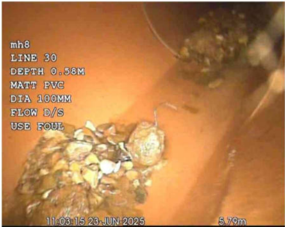
MH 8X_38f1dedd-0636-48cb-bb58-a64c45474d27_20250701_170733_833.jpg, 00:00:20, 5.79 m Finish node, major connection without manhole, reference: L30
