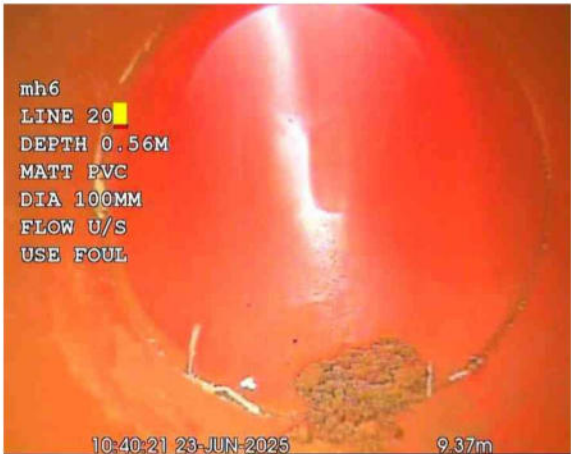
L20X_ffd22232-8f7c-43a1-9452-a7ba47932ba9_20250701_17 0139_418.jpg, 00:00:26, 9.37 m Line deviates up
