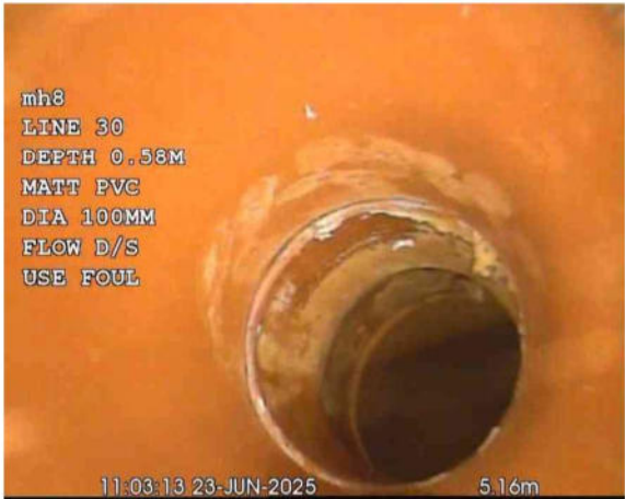
MH 8X_ea9f699c-a617-46f3-b323-6ab1b76fb2e4_20250701_170732_567.jpg, 00:00:18, 5.16 m Line deviates down
