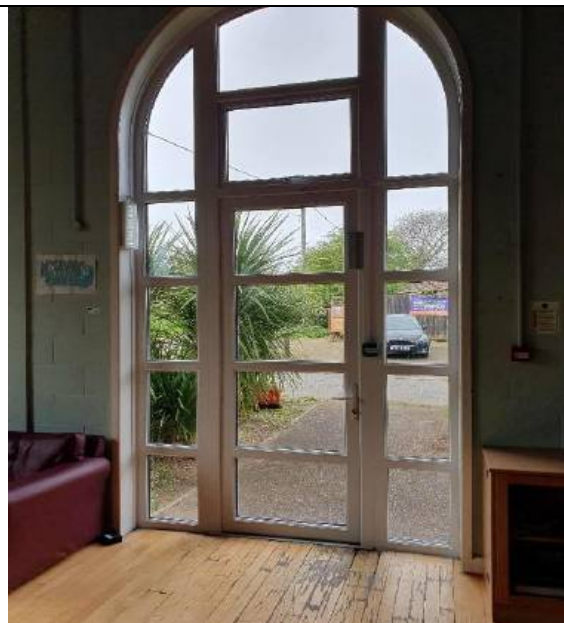
Photograph 2: Internal area of B1 with uPVC door to the western elevation and water damage to the flooring.
