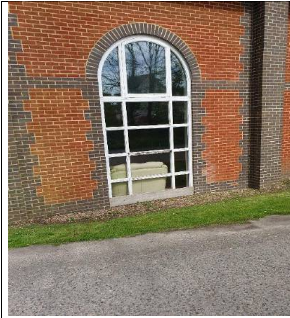
Photograph 5: External southern elevation of B1 with damage to the wooden window frame.
