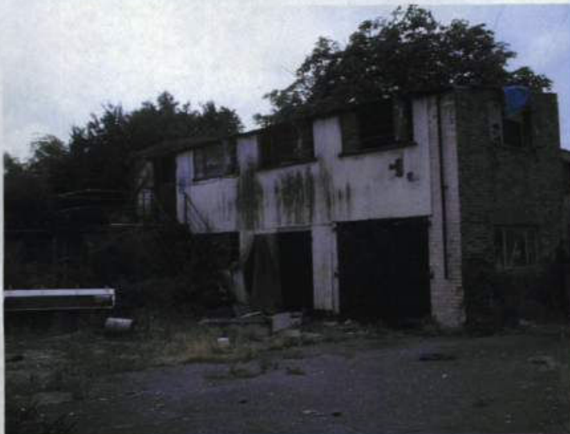
One of the existing out-buildings now derelict, having been vandalised and squatted in, it is now burnt out.
