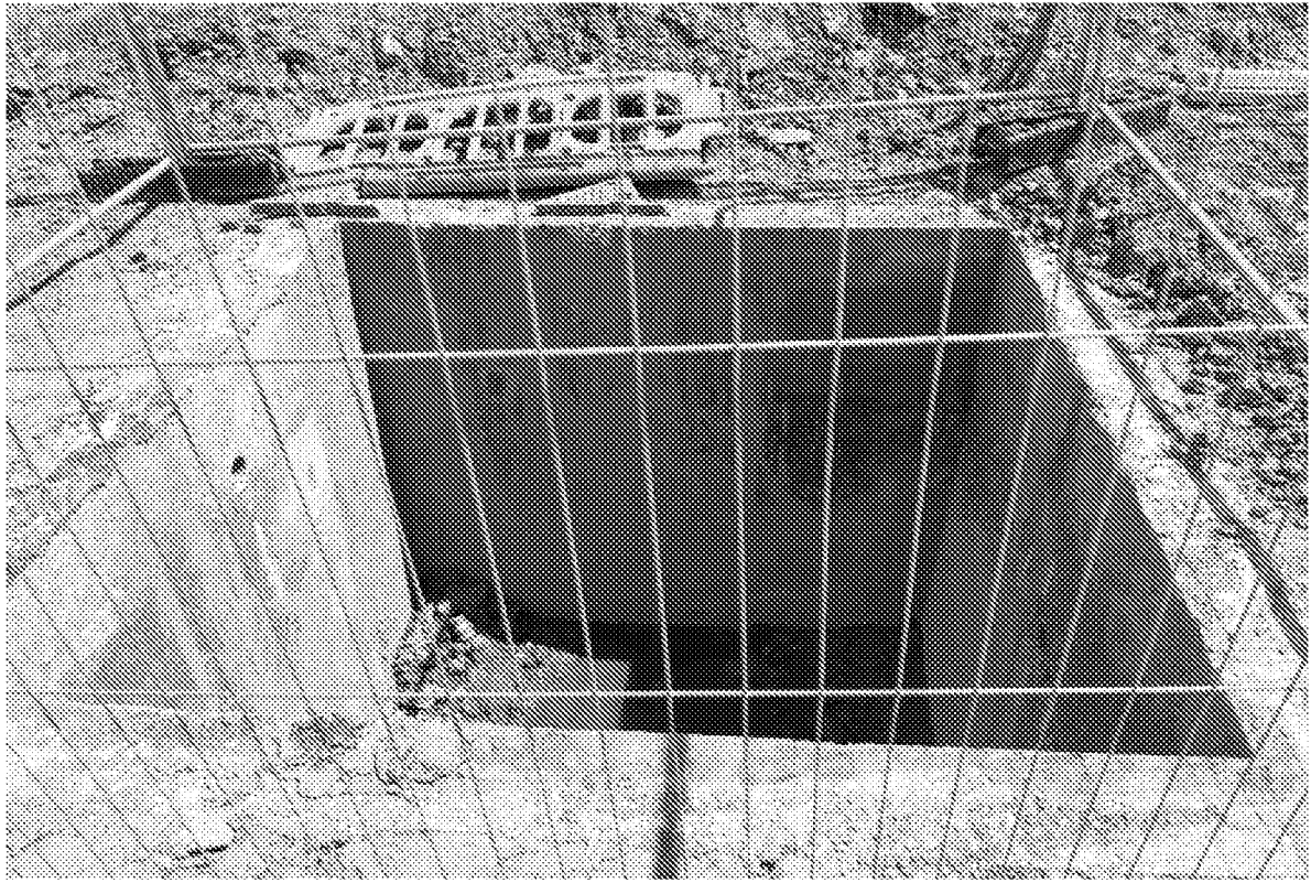
Plate 5 21st May 2019 - Cesspit located on plot 2 still visible on this visit.
