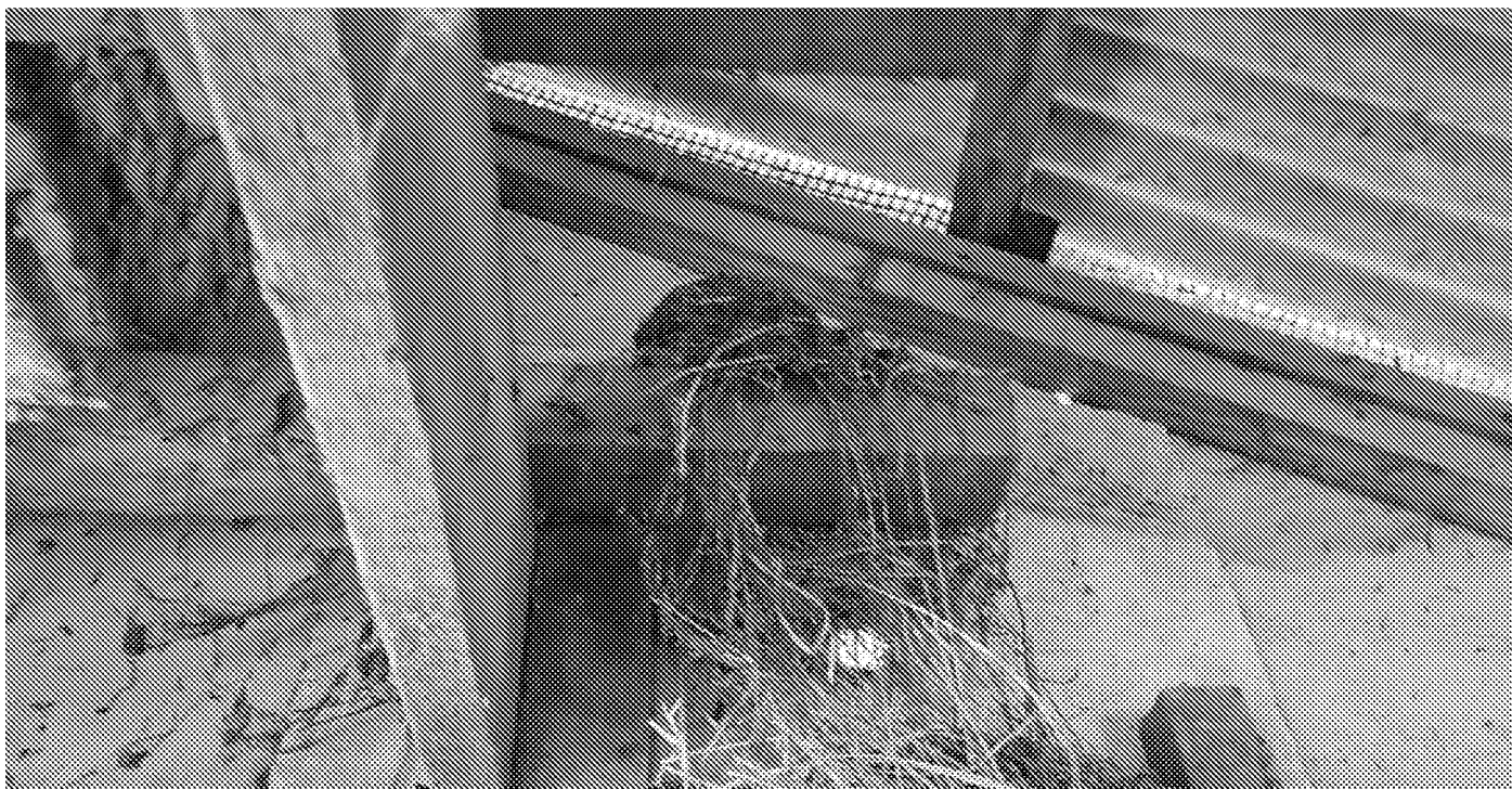
Photograph No. 5 - Disused bird nest located within Building B2.
