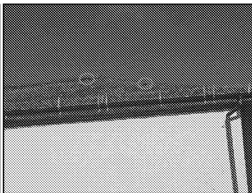
Figure 6: Gaps in roof tiles in 2019
