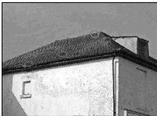
Figure 5: Gaps in roof tiles in 2016
