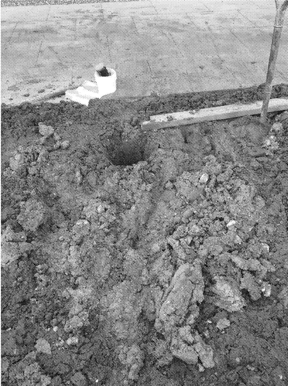
Photo of hole with tape in place
