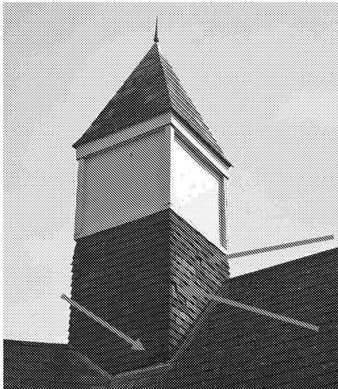
Plate 6 - Gaps present amongst the clay hanging tiles on the clock tower.
