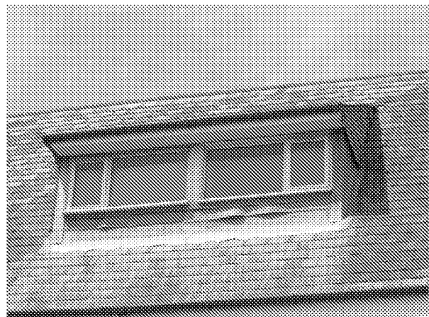
Lifted lead flashing around windows
