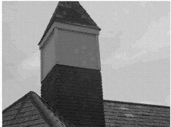
Clock tower, western aspect, missing/slipped hanging tiles
