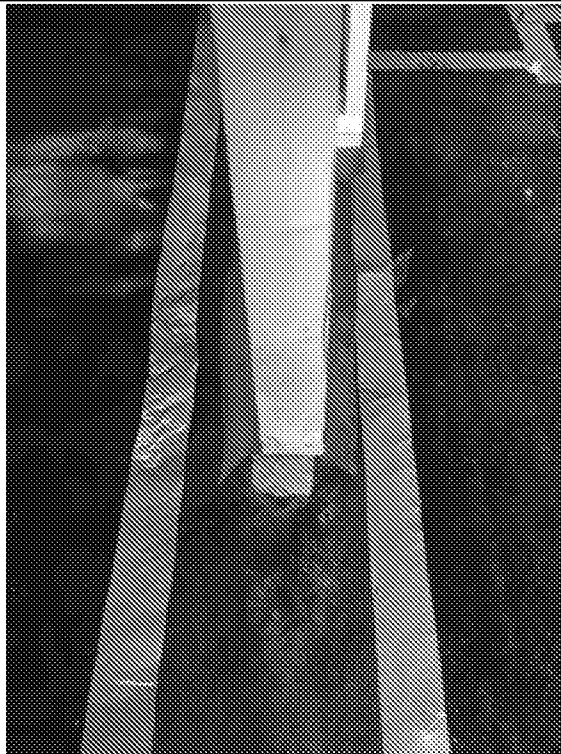
Photograph 13 – Plots 1-2: Example of Detailing Through Doorway with Membrane Under Internal Wall
