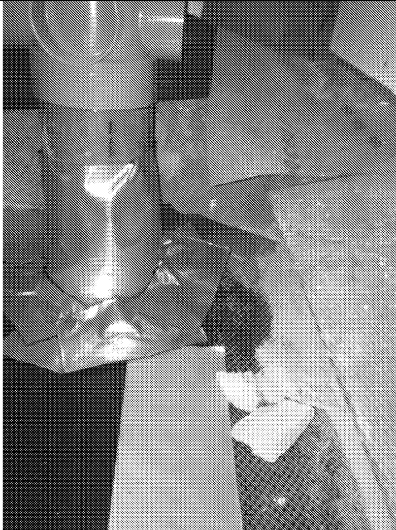
Photograph 23 – Defect in membrane installation
