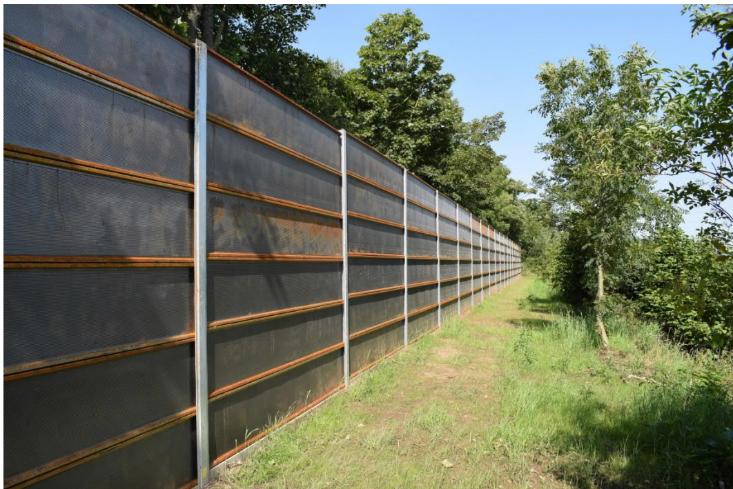
M6 near Carlisle – Before steel has weathered
