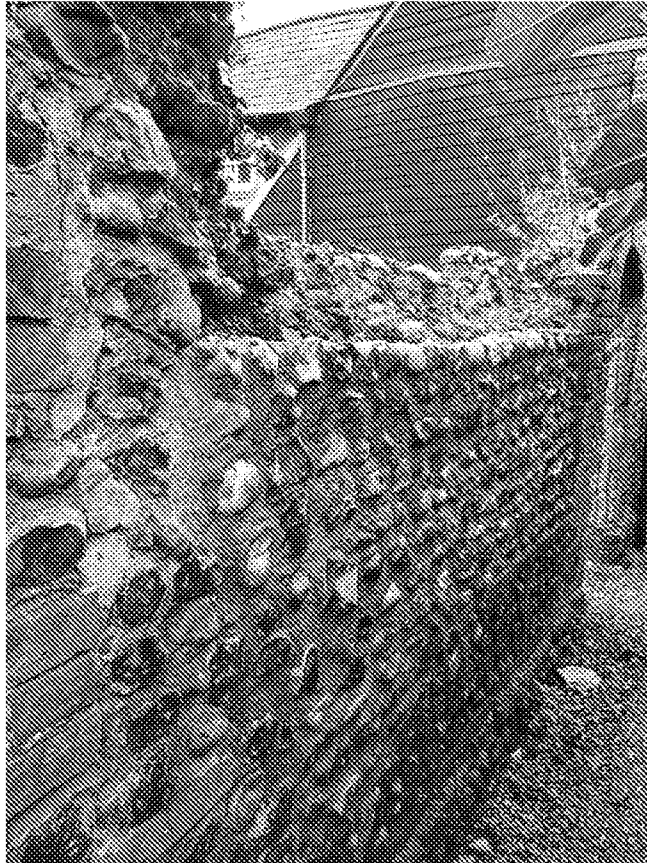
Badly re-built areas of the external wall, to be taken down and re-built
